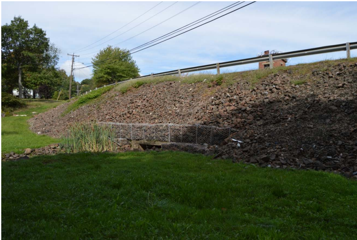
Photo 8d – A panoramic view of the central and right side downstream embankment, in good and stable condition in 2016.
