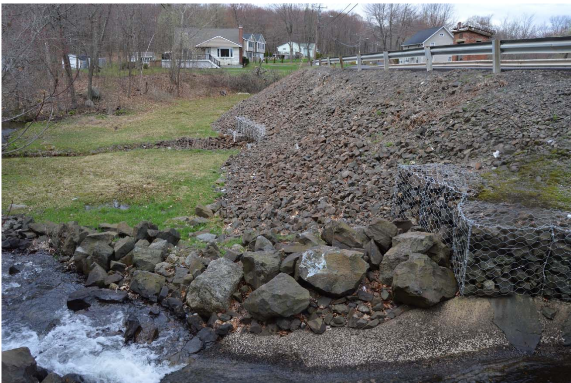
Photo 2b – The downstream side of Cedar Lake Dam, as seen from the left downstream abutment area. The spillway discharge channel is in the foreground.
