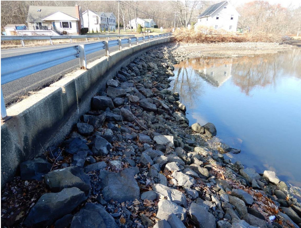
Photo 3c – Riprap lining the upstream embankment slope on the right side of the gatehouse, during the annual winter drawdown.
