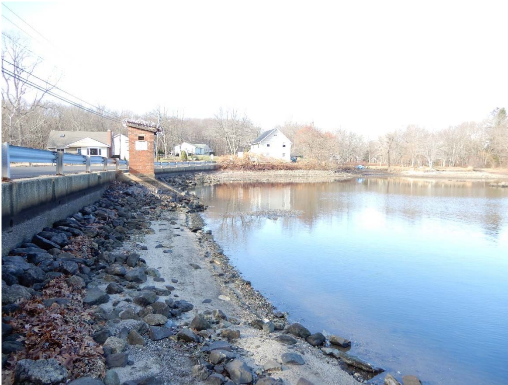
Photo 1d – An overview of Cedar Lake Dam, again as seen from the left side upstream abutment, this time during the winter drawdown period. The riprap apron in the foreground and along the upstream slope is in satisfactory condition.
