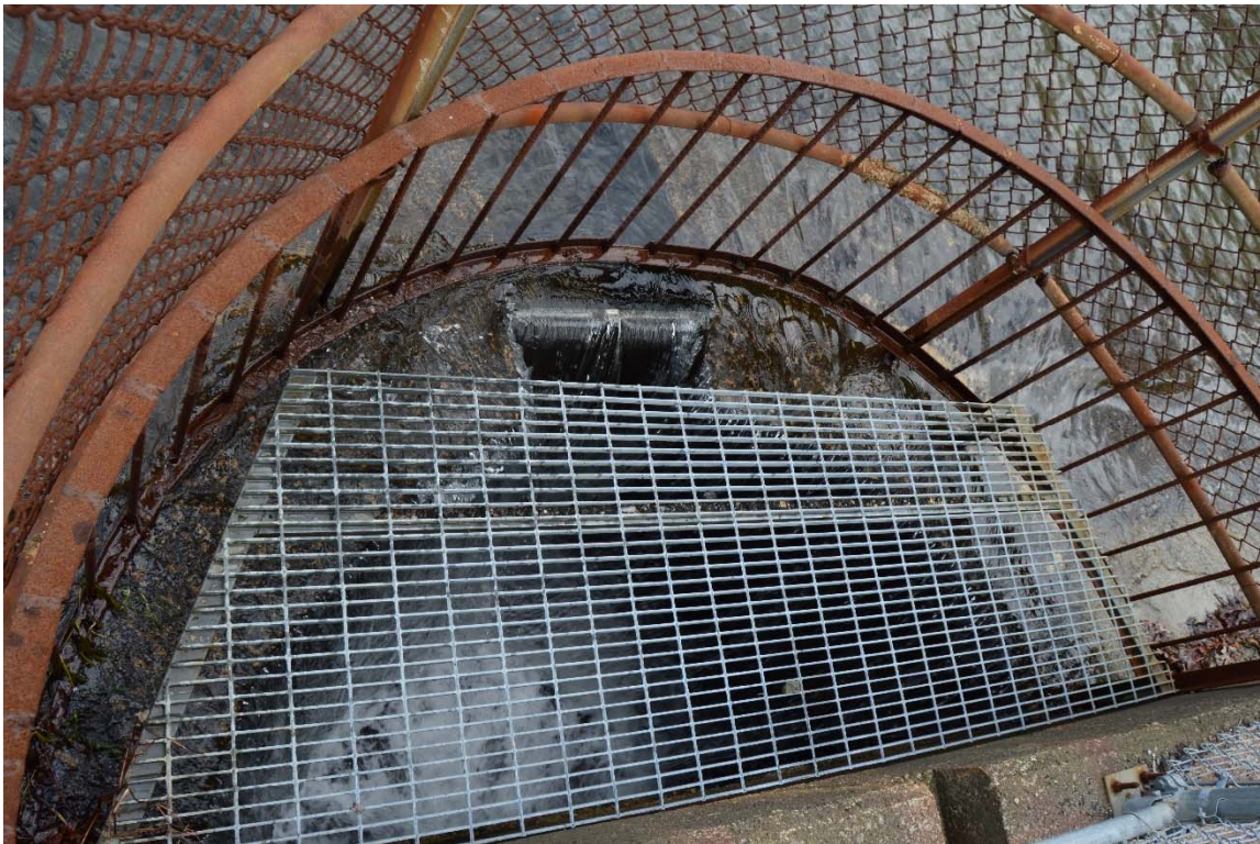
Photo 10a – A view of the spillway as seen from the immediate downstream (looking downward from the adjacent roadway).
