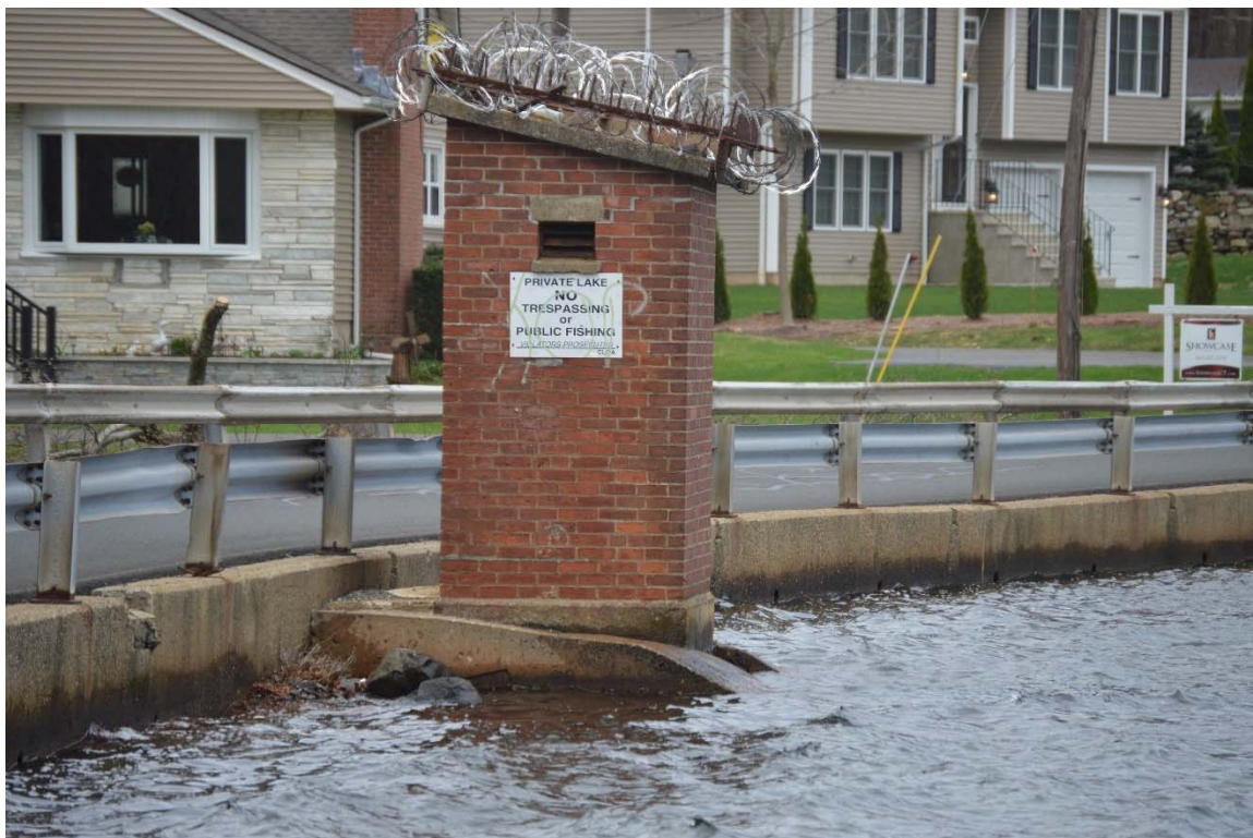
Photo 16e – An overview of the gatehouse as seen from the left upstream side.
