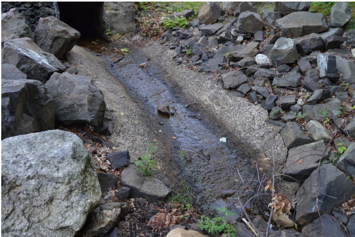
Photo 14d – The spillway chute discharge, at the exit of the tunnel area beneath North Street, with riprap side slopes.
