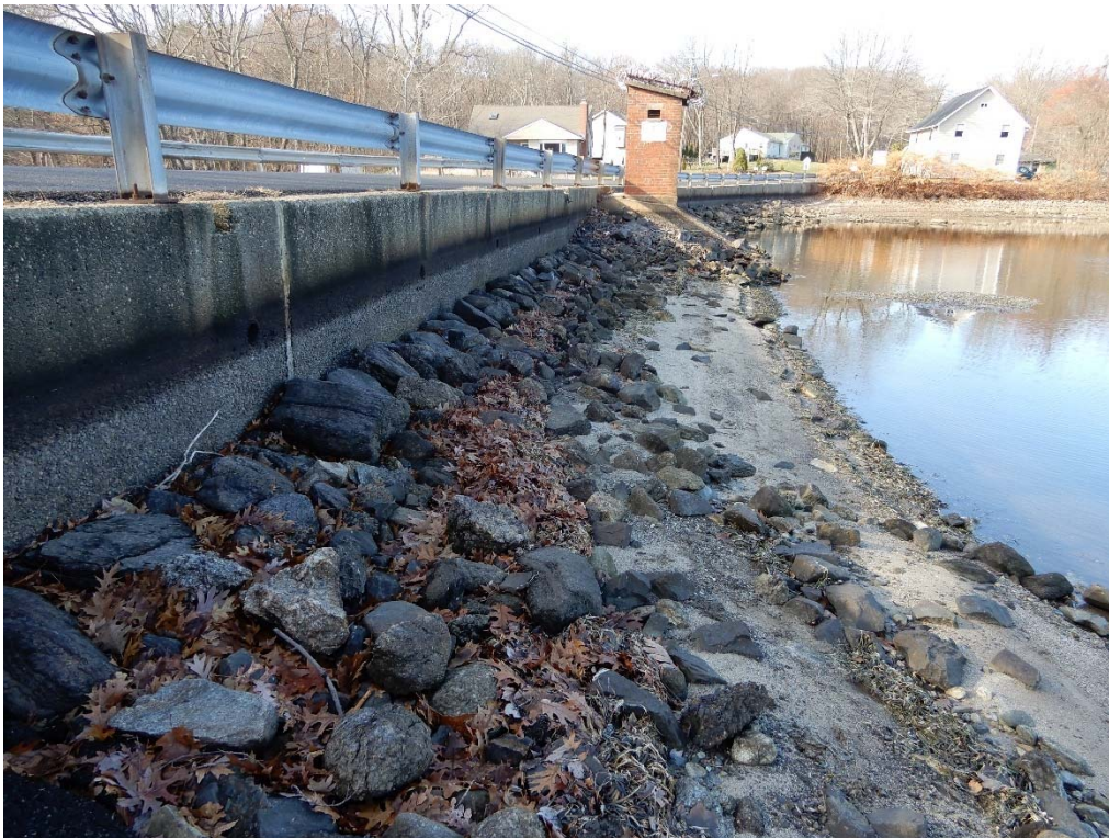
Photo 4h – Looking back along the upstream embankment toward the gatehouse during the winter drawdown.
