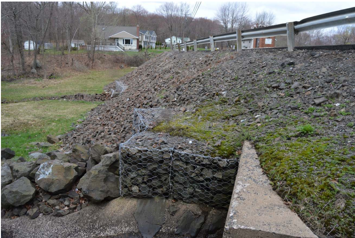
Photo 8c – A sweeping view of the downstream embankment face, taken from the discharge channel outlet.
