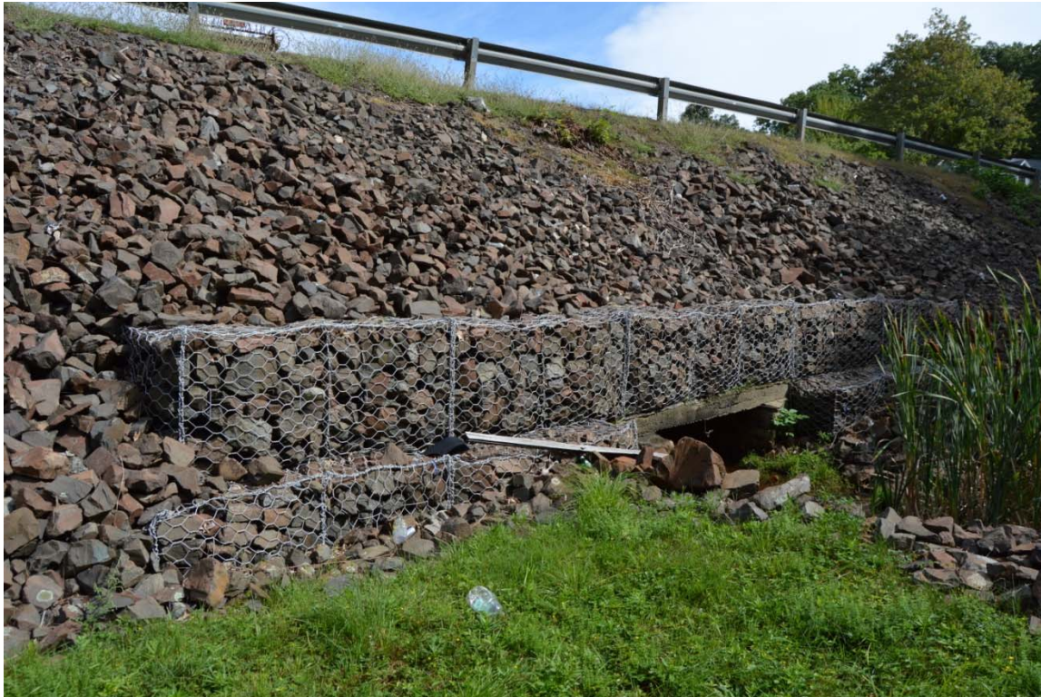
Photo 7g – The central section of the downstream embankment. The stone cover is stable in this area (note the gabion metal mesh cages placed to prevent sloughing of embankment stones).
