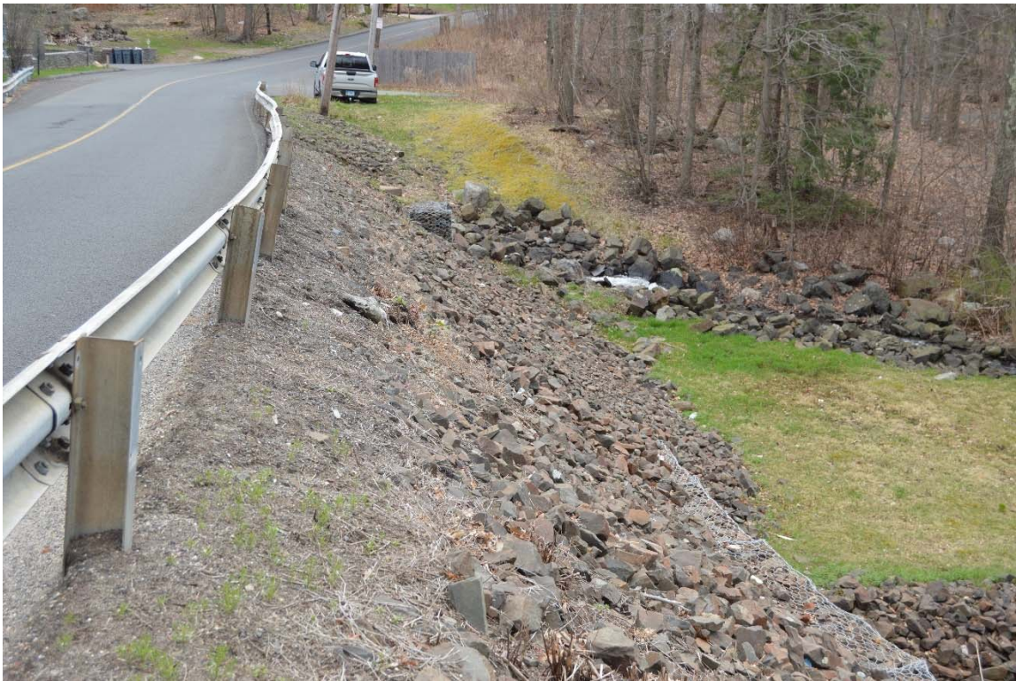
Photo 7c – The stone-lined face of the downstream embankment. This area has been maintained clear of vegetative growth between the stones. The discharge channel at the right-center of the photo emanates from the spillway.
