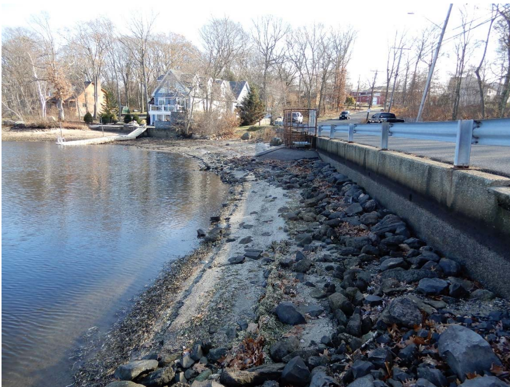
Photo 4f – An overview of the central section of the upstream embankment; the spillway is visible in the center of the photo.
