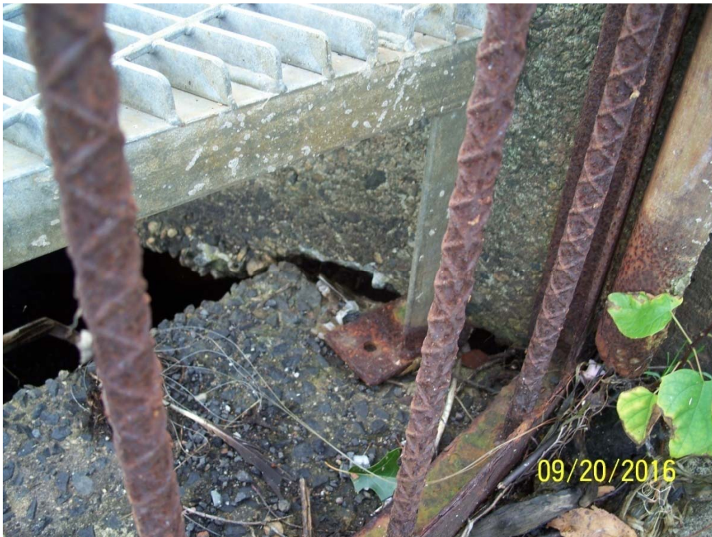
Photo 21j – The right side of the spillway at the junction between the weir and right side abutment wall. Note the gap between concrete wall sections. This should be cleaned and mortared. Wear of the steel bars and the bracket for the protective outer grate is also extant.
