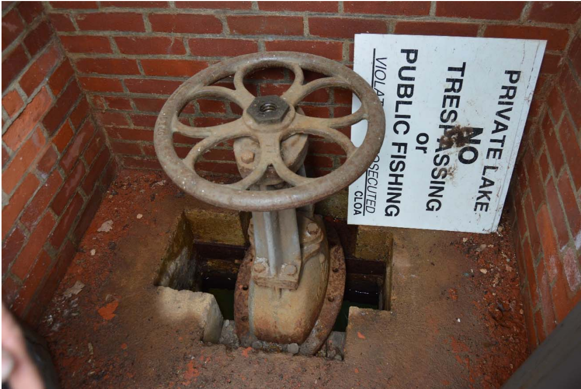
Photo 21a – The interior base of the gatehouse. Note the mild corrosion on the base brackets for the valve operator, which should be cleaned and coated. In addition, the occasional difficulty in turning the valve indicates that the valve needs to be serviced on a regular basis (i.e., bonnet removed, gaskets replaced, stuffing repacked, etc.).
