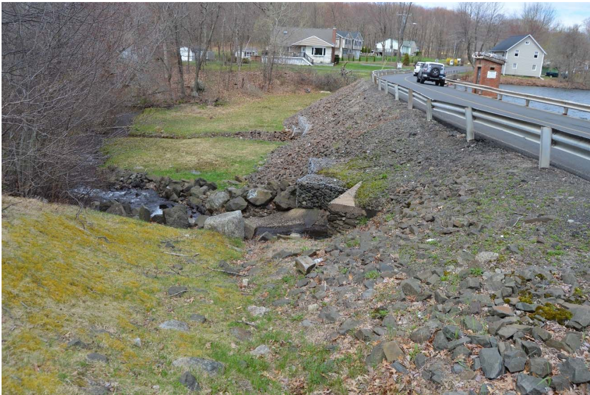
Photo 2a – An overview of Cedar Lake Dam, as seen from the left downstream abutment area.
