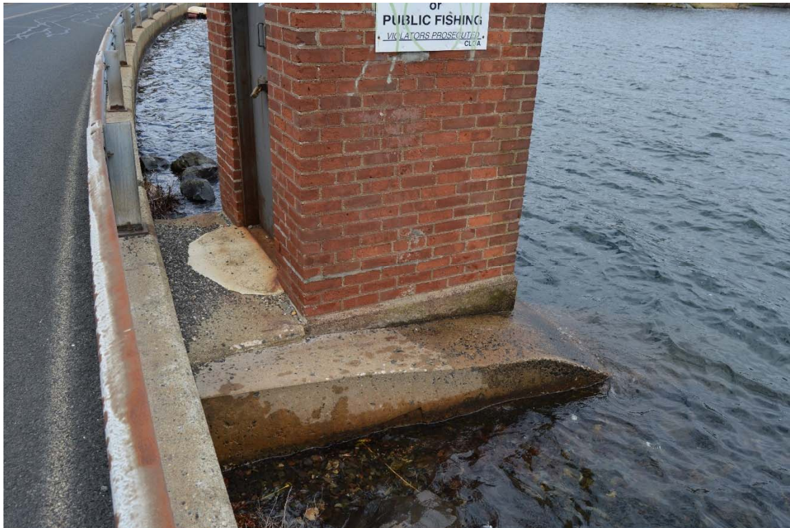
Photo 16d – The left side of the gatehouse and foundation, in a similar condition to the right side.
