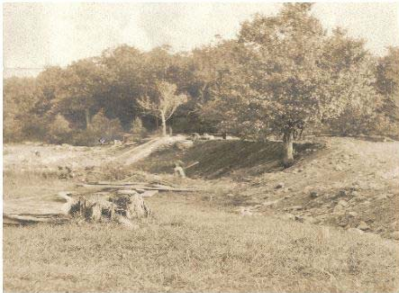
Oct. 14, 1907, MR Cedar Swamp dam, in process of raising, raising road and widening earthen embankment on water side.
