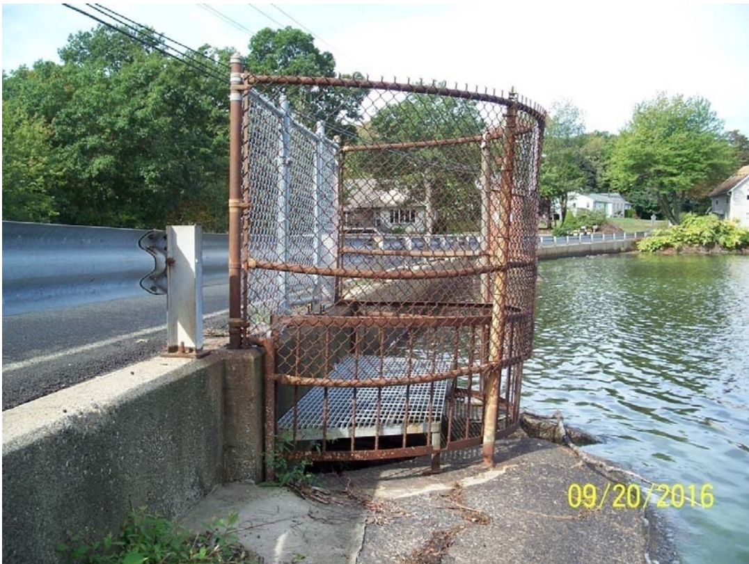
Photo 9e – The spillway and appurtenances as seen from the left side looking westward at a lower flow period in 2016. Note the concrete approach pad on the left side.
