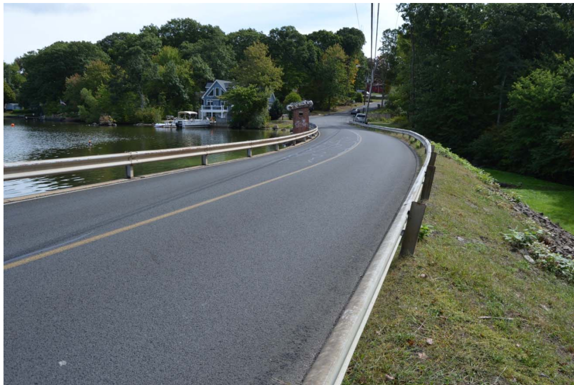
Photo 5b – An overall view of the dam crest, formed by North Street, as seen from the right abutment in 2016. The gatehouse on the upstream side is situated in the center of the photo.
