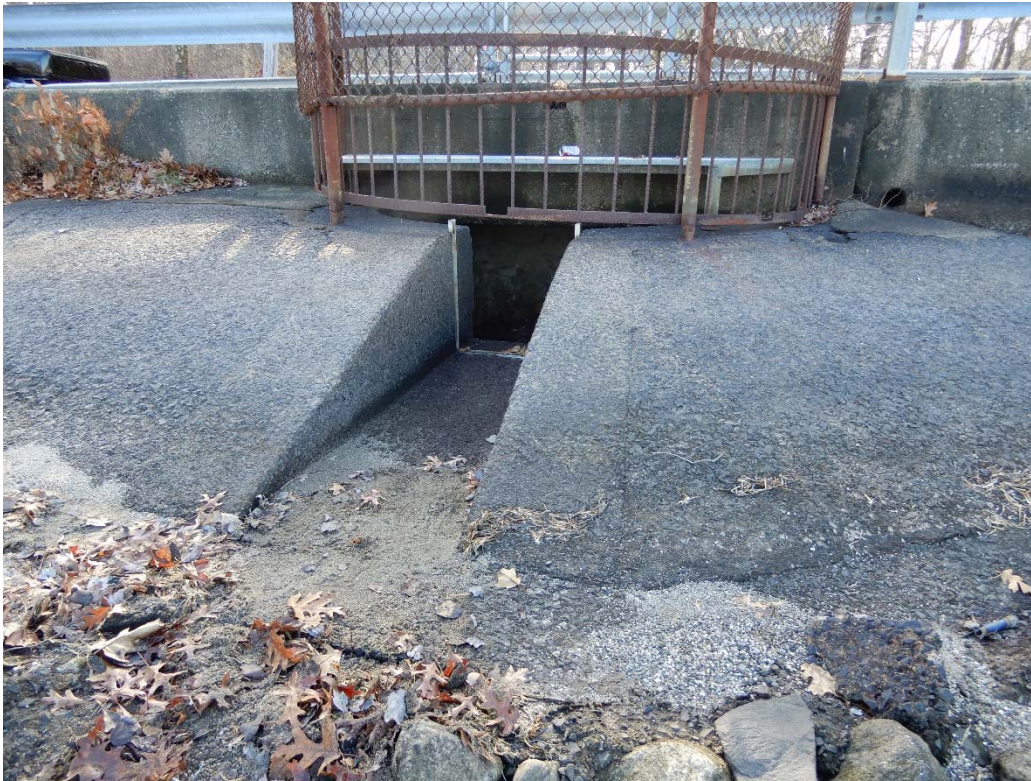
Photo 9f – The spillway approach area as seen from the upstream during the winter drawdown. The concrete is in overall good condition with minor spalls and cracks near the overflow crest area.
