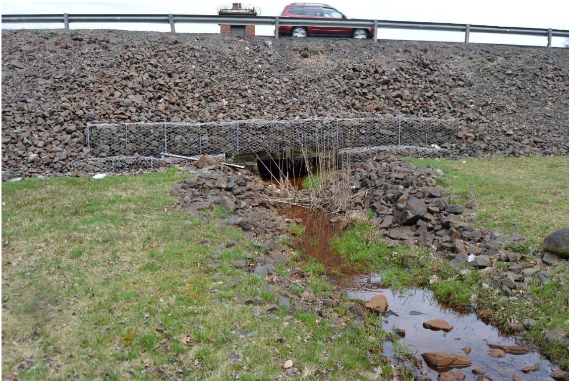
Photo 14a – An overview of the stilling basin at the low level outlet discharge.
