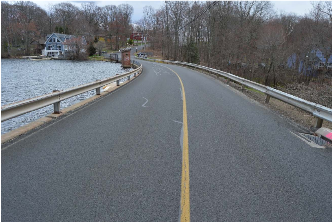
Photo 5a – The crest of Cedar Lake Dam, as seen from the right abutment.
