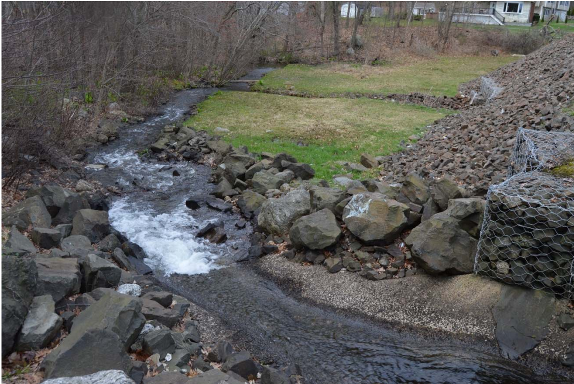
Photo 14c – The concrete splash pad at the main spillway discharge outlet, with riprap lined channel and side slopes extending further downstream.
