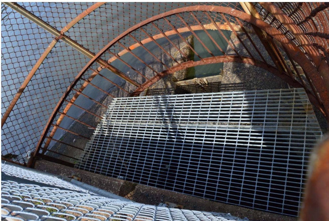
Photos 11 & 12 – A view of the concrete approach apron and adjustable weir channel surrounding the spillway inlet area. The concrete is a bit weathered but still in sound condition.
