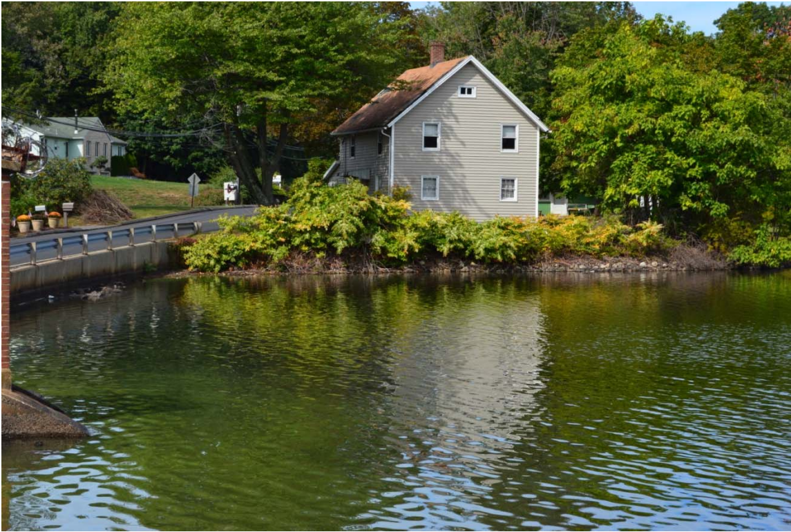
Photo 21g – Another view of the right side upstream embankment area of Cedar Lake Dam, with the full extent of seasonal brush growth visible (2016 photo).
