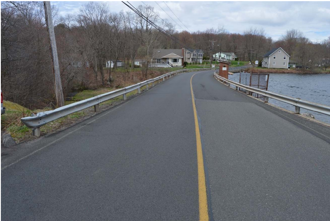
Photo 6a – The crest of the dam as seen from the left abutment.
