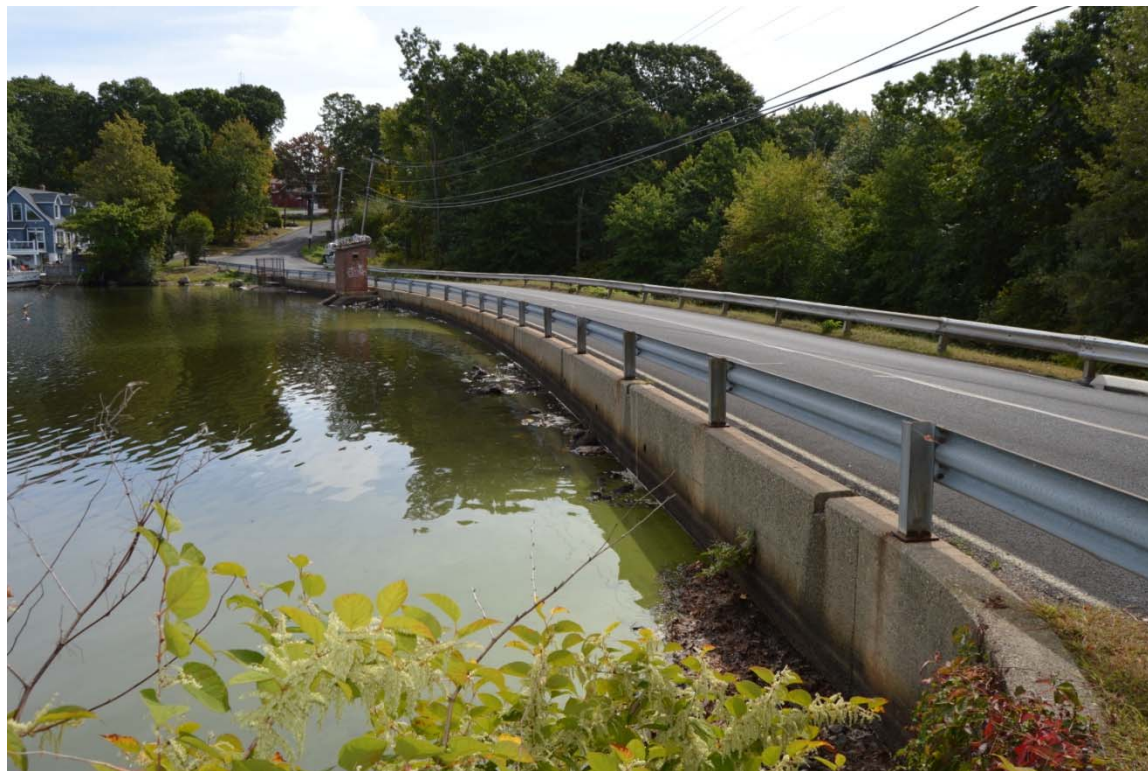
Photo 3b – The upstream face of Cedar Lake Dam, as seen from the right upstream end of the dam during a low water level period in 2016.
