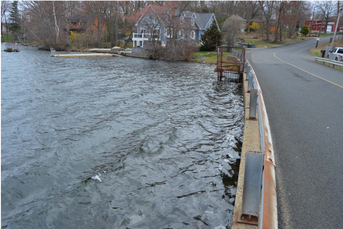
Photo 4c – Looking eastward toward the left upstream end of the dam from the left side of the gatehouse.
