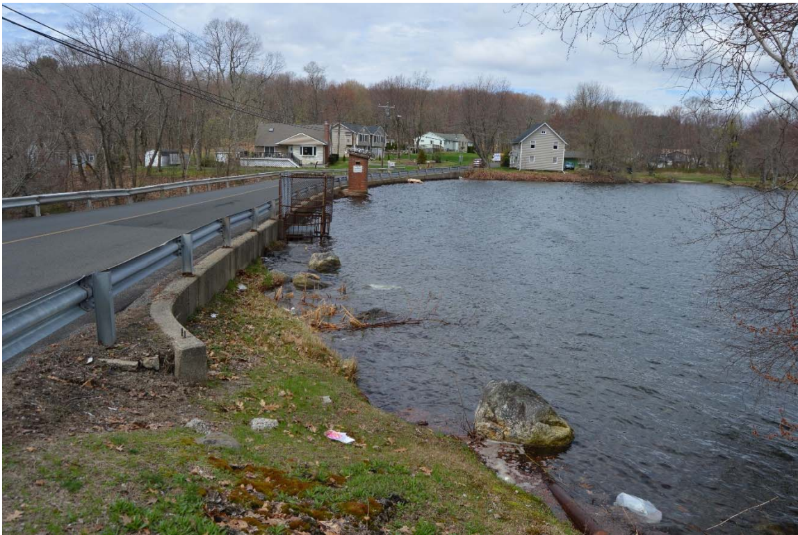
Photo 4a – A view of the upstream face of the dam, seen from the left upstream abutment area.
