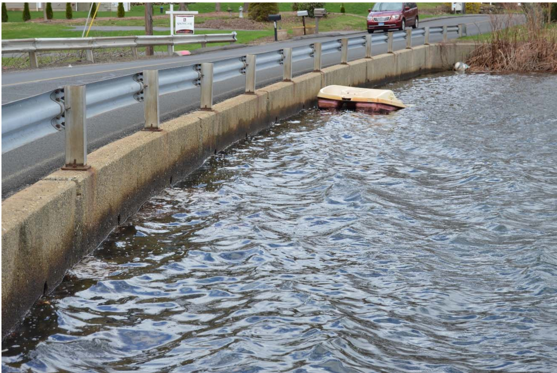
Photo 4d – The right upstream side of the dam, as seen from the left looking right. The concrete retaining wall is generally in good, stable condition here and along the breadth of the upstream side.
