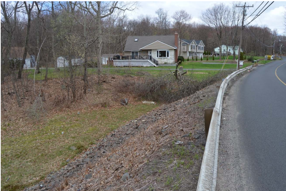
Photo 7b – Looking westward toward the right downstream end of the dam embankment.
