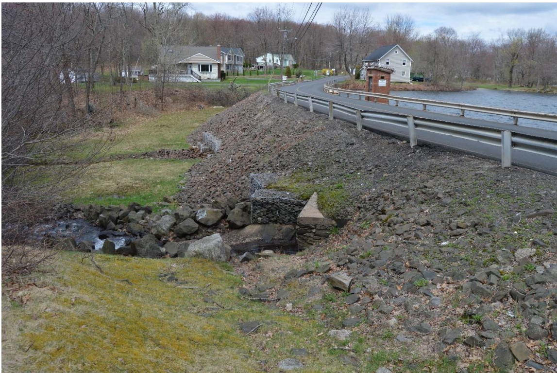
Photo 8a – An overview of the downstream face of the dam, as seen from the left abutment. Again, the spillway discharge channel is in the foreground.
