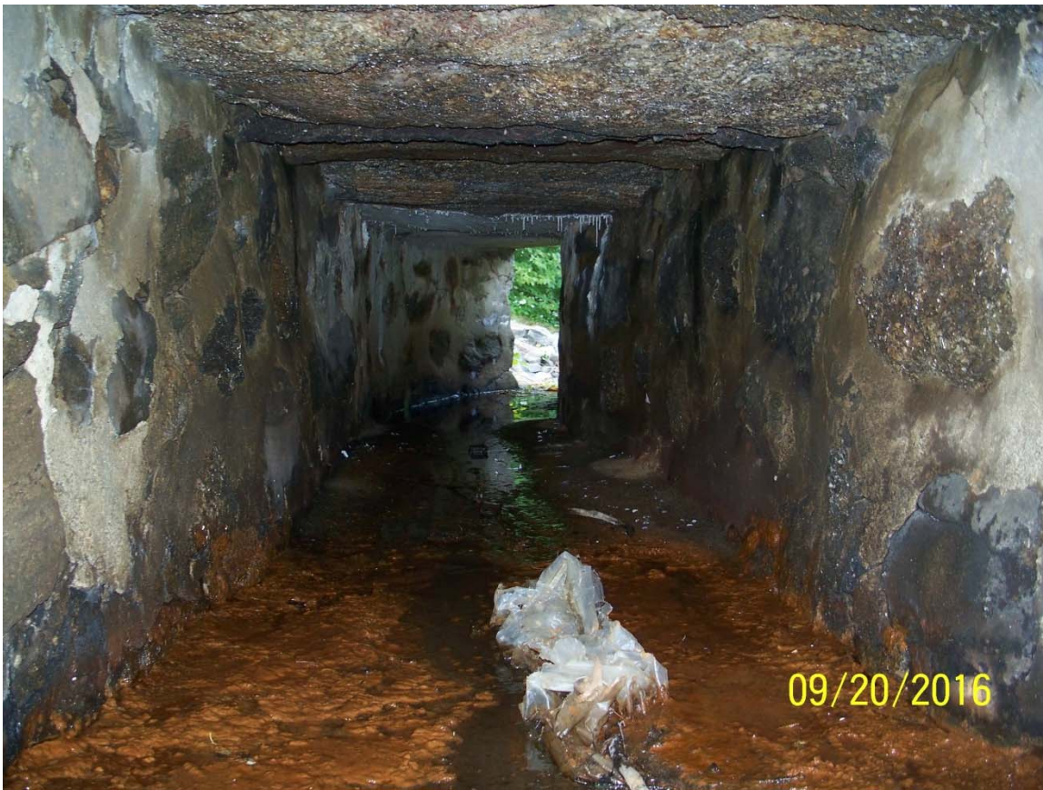
Photo 21d – The interior of the spillway tunnel (looking downstream from the upstream end), showing a section of roof with open voids between stone that spans the width of the tunnel.
