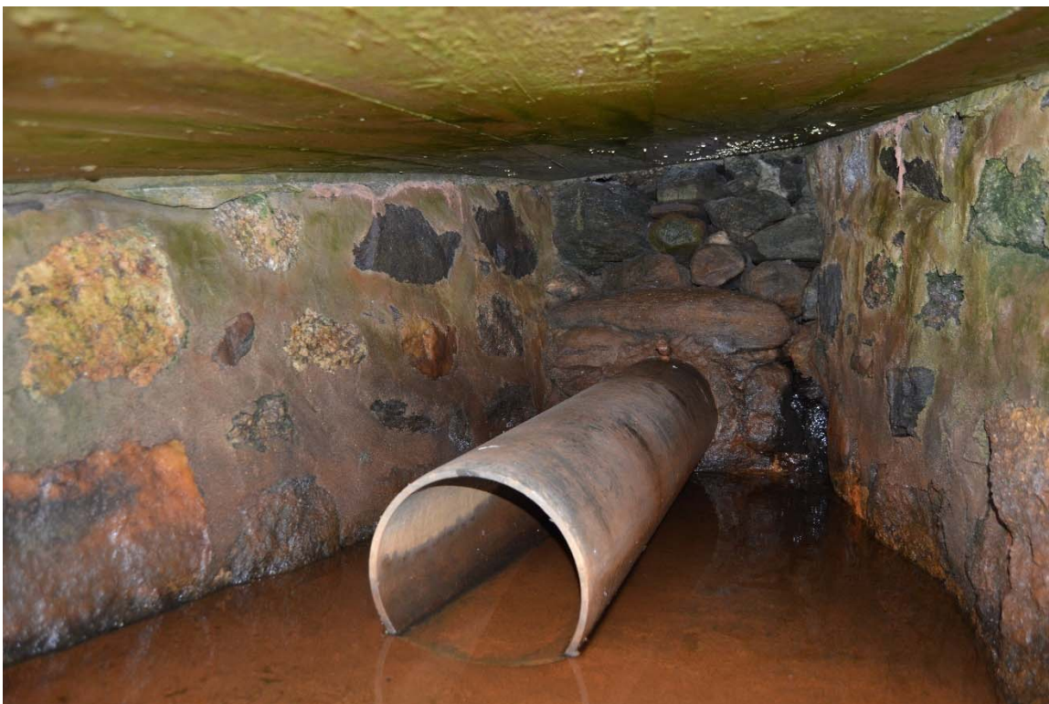
Photo 19b – A head-on view of the low level outlet pipe discharge. The coupling or connection fitting with the remaining outlet pipe is unknown.
