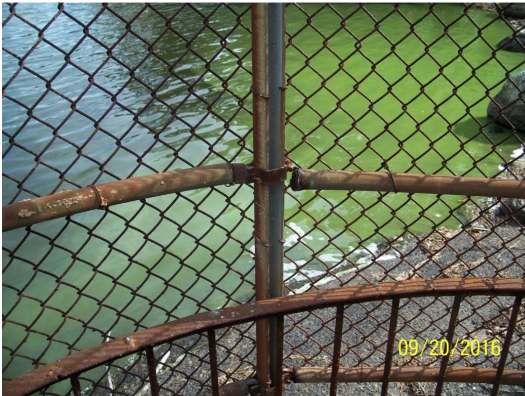
Photo 21h – The fencing surrounding the spillway inlet has begun to show wear, along with separation of some structural members. Steel should be cleaned and coated where practicable, while deteriorated portions of the chain link fence should be replaced.
