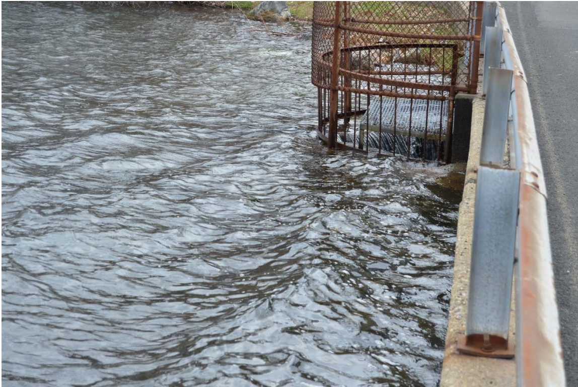
Photo 9b – Looking at the spillway from its right side. There was substantial flow on the date of the first inspection.
