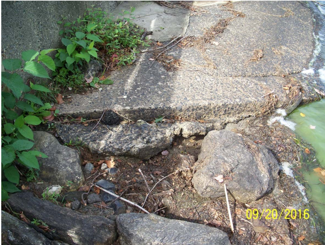
Photo 21i – Concrete deterioration at the left upper end of the spillway approach slab. The concrete must be cleaned, and cracks and openings closed off and re-mortared where necessary.
