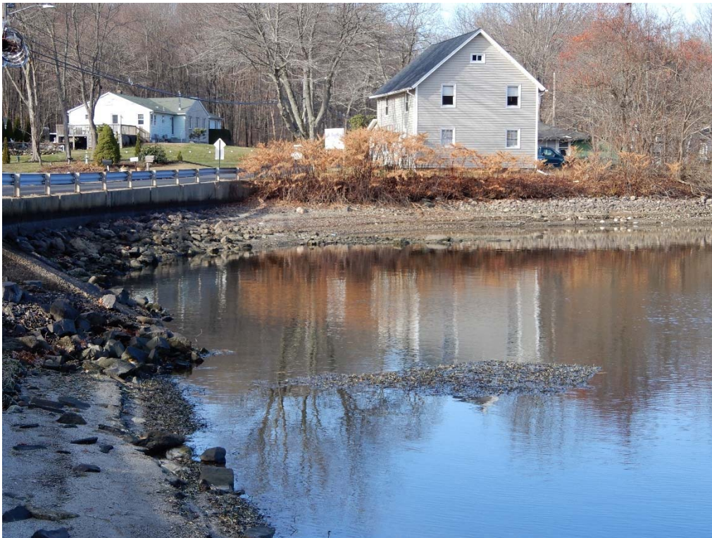
Photo 3d – The right end of the upstream embankment during the winter period, again in satisfactory condition. The intake training wall at the gatehouse can be seen at the center-left of the photo.
