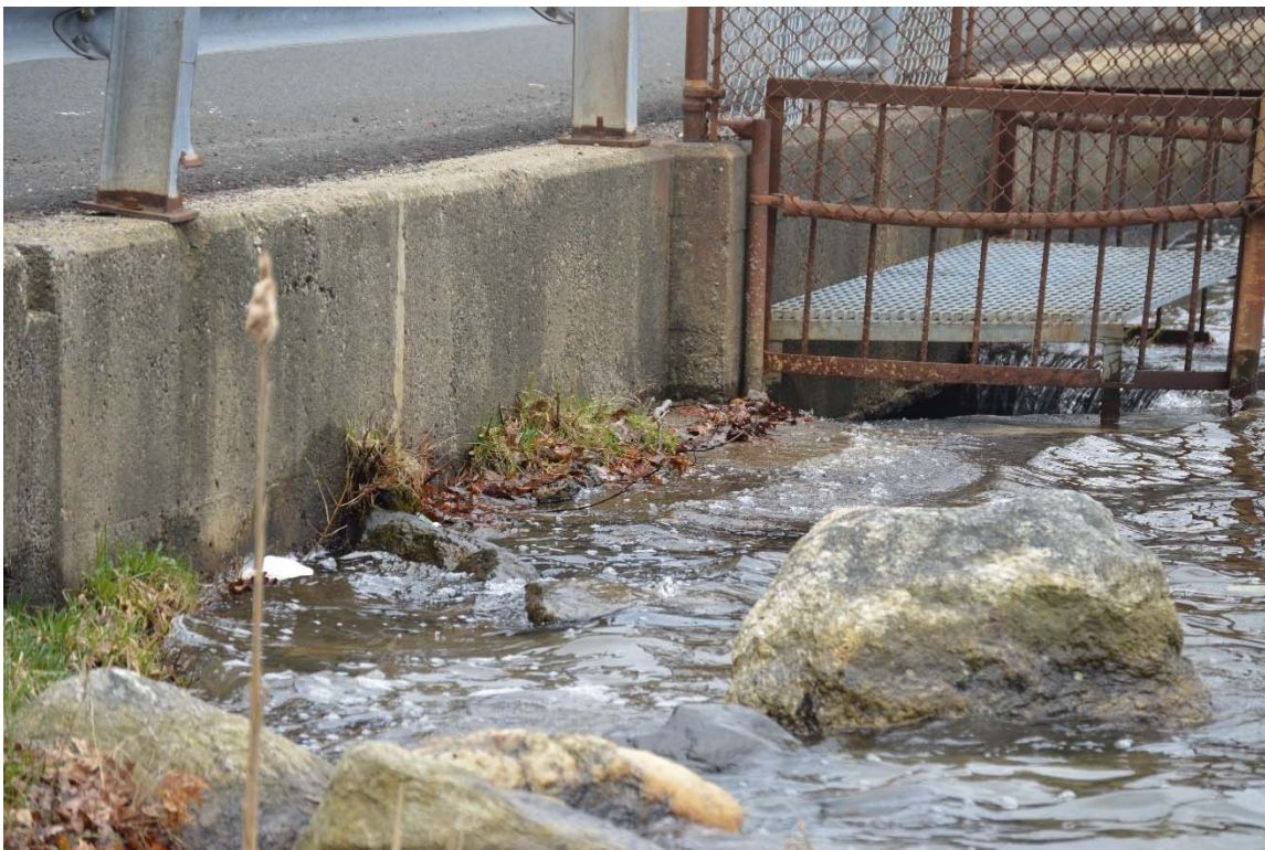
Photo 21f – The left side of the spillway approach area, showing the corrosion present on the fence post and rails surrounding the spillway.
