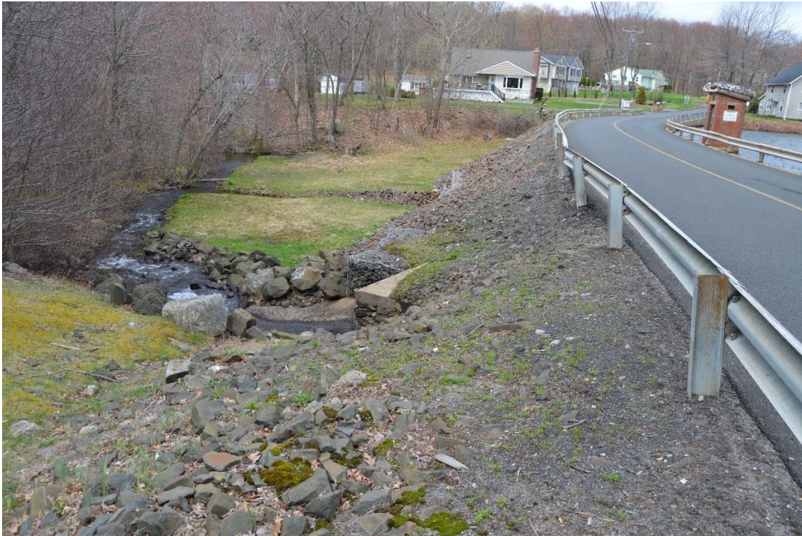
Photo 15a – An overview of the downstream area, with the downstream spillway channel and its junction with the low level discharge channel visible in the left center of the photo.
