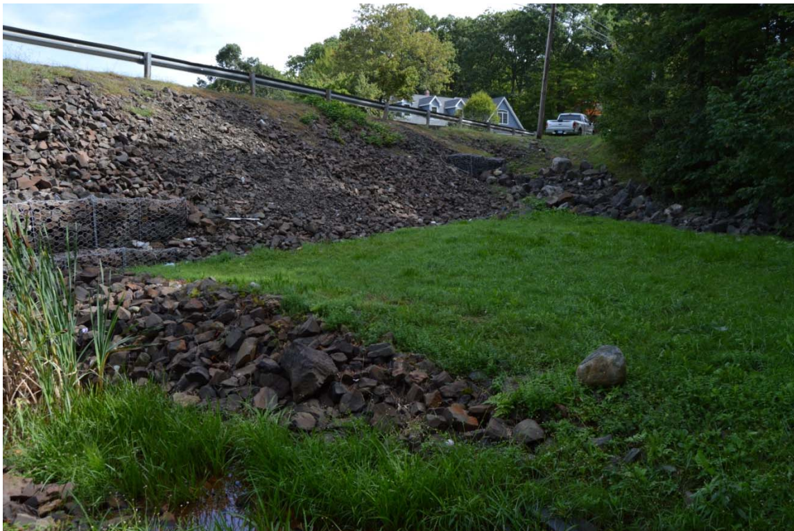
Photo 7f – Looking eastward from the center of the dam for an overview of the left half of the downstream embankment. The riprap lined low level outlet discharge channel is in the left foreground of the photo.
