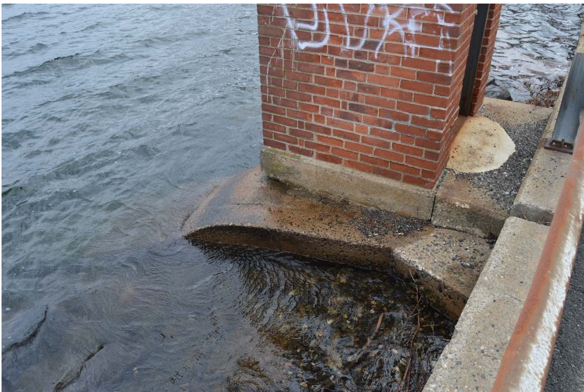
Photo 16c – Again taken from the right side, this close up view shows the foundation of the gatehouse sitting atop the inlet channel sidewalls. The concrete is in sound condition.
