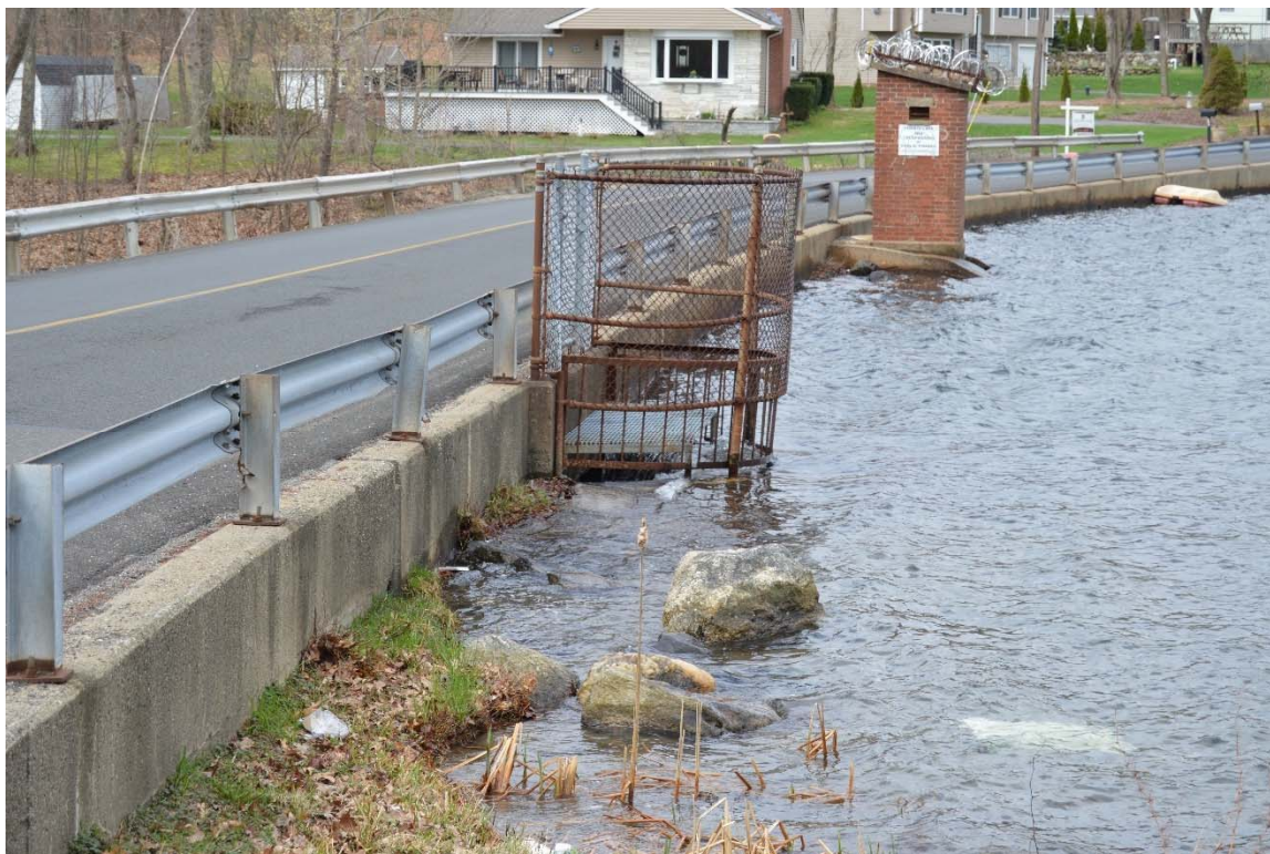
Photo 9a – An overview of the spillway and its approach area, as seen from the left side.
