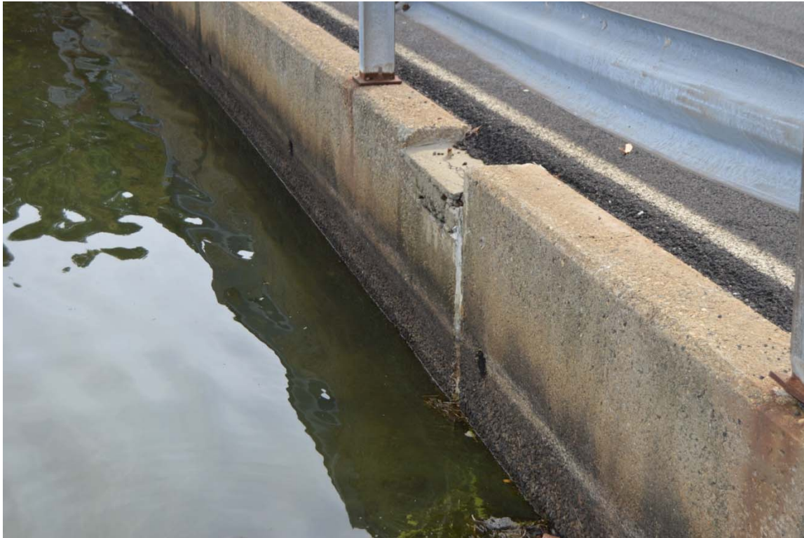
Photo 21m – A leak off for road drainage to flow into the lake. Note minor concrete deterioration just below the leak off point. This area should be patched and coated before the deterioration worsens.
