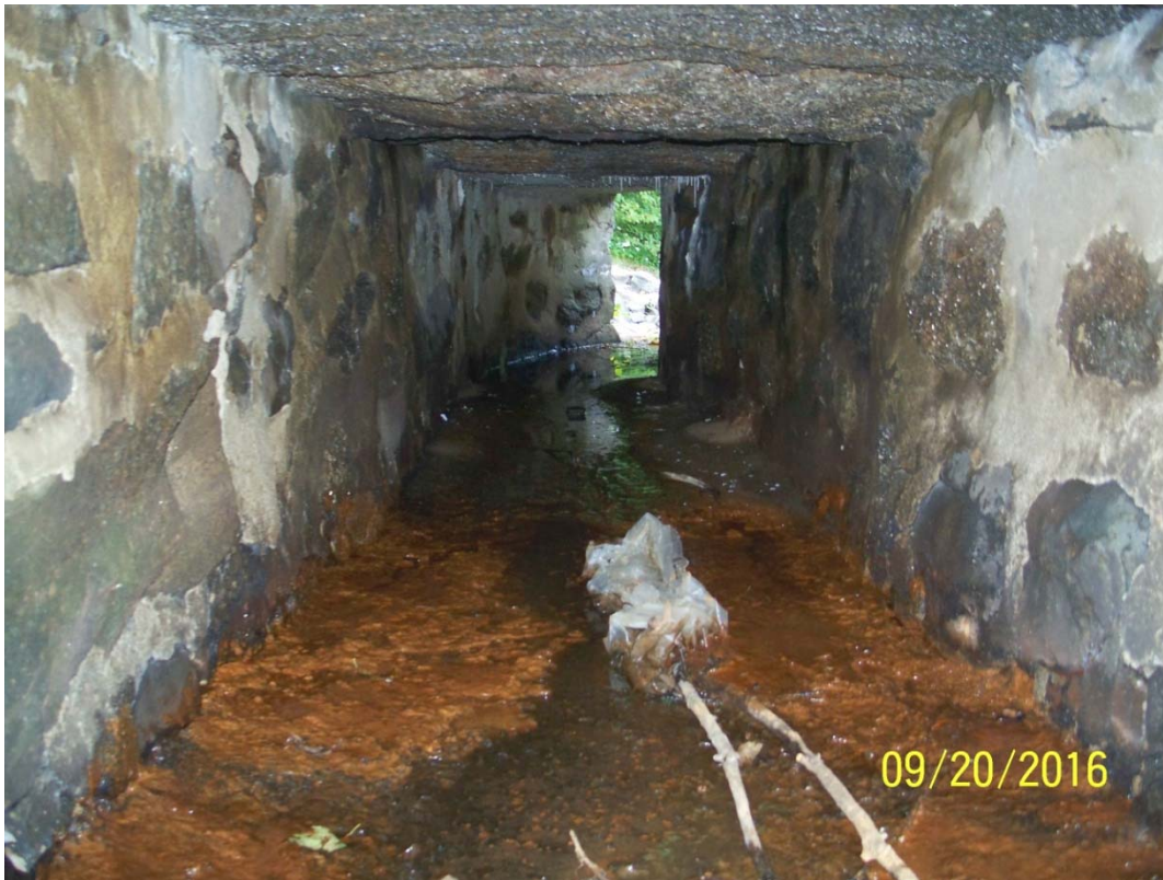
Photo 19e – The upstream section of the spillway discharge channel, which runs under North Street, as seen in 2016 from the upstream end. Note the roof in this area is open stone masonry – slabs spanning its width.
