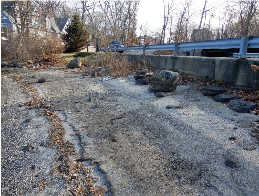
Photo 4g – The upstream embankment slope to the left of the spillway. The concrete wall here is in stable condition.
