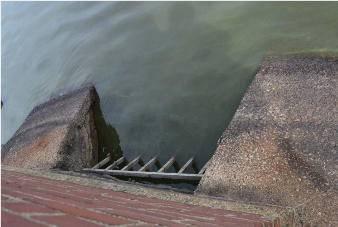
Photo 19g – The intake for the low level outlet pipe on the upstream side of the gatehouse. The trash rack covering the opening appears to be in good condition judging from the visible portion above water level.
