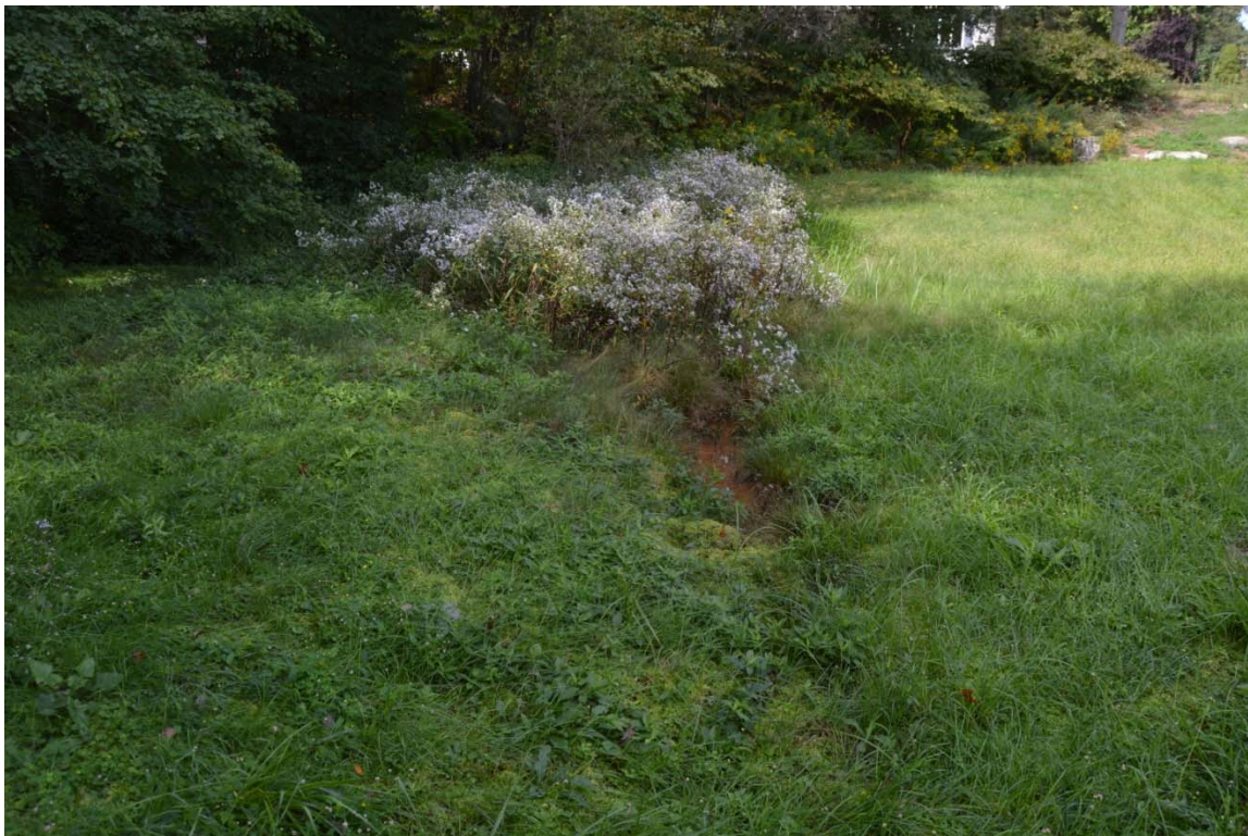
Photo 21n – An area of standing water near the base of the downstream slope, indicating seepage through the embankment, although to a moderate extent. Continued monitoring is recommended.
