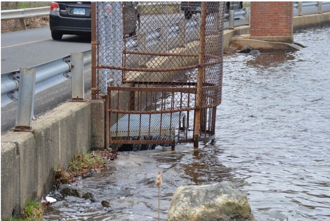
Photo 9c – A closer view of the spillway from the left side, with the trash rack visible. The rack is in good condition, but the fencing around the spillway exhibits progressive corrosion.
