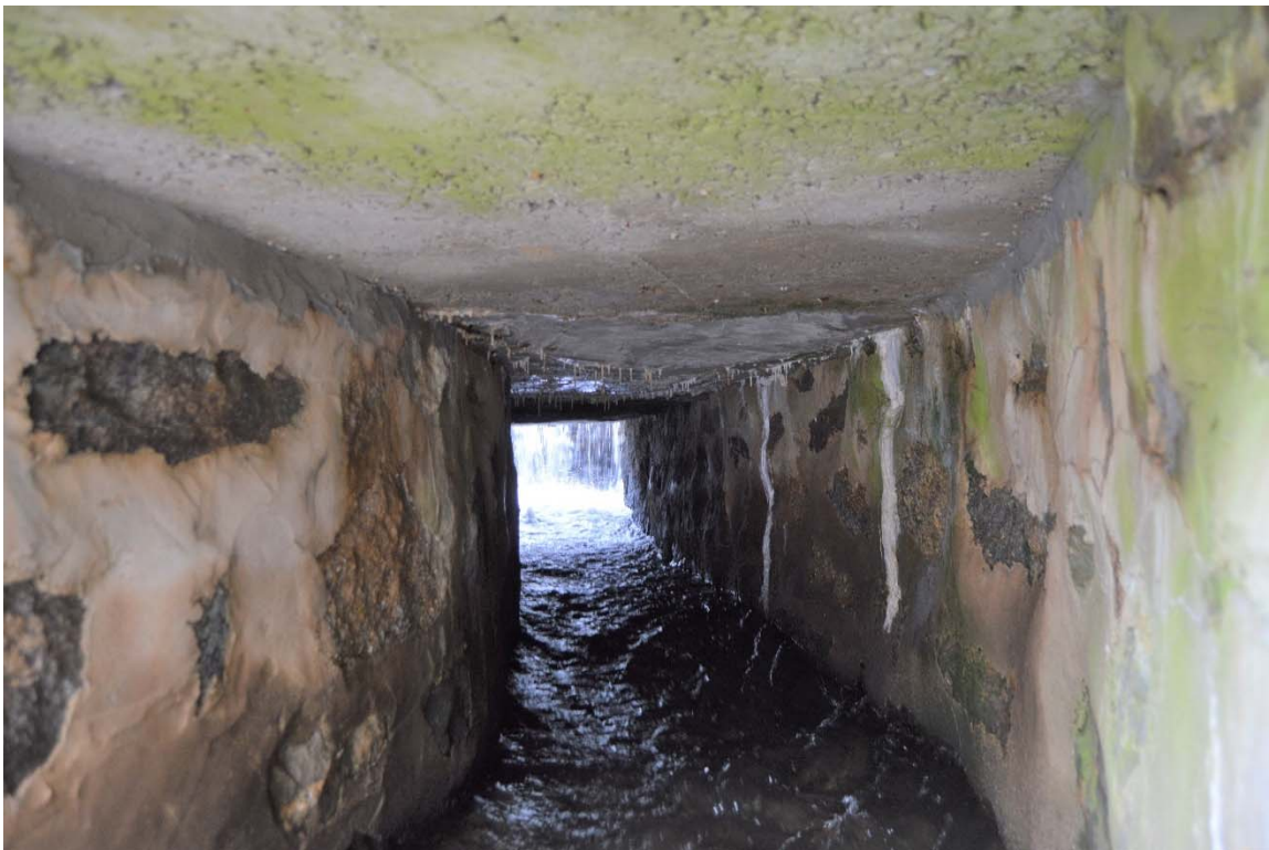
Photo 19d – Progressing upstream through the spillway discharge tunnel. The masonry sides of the tunnel are covered with a cementitious coating; the roof appears to have been cast rather than coated. The concrete roof extends only halfway up the tunnel from the downstream end; the rest is open stone – see Photo 19e.
