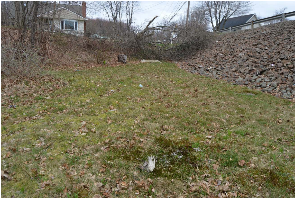
Photo 7e – The right end of the downstream embankment and toe area. The downed tree at the abutment has been removed.
