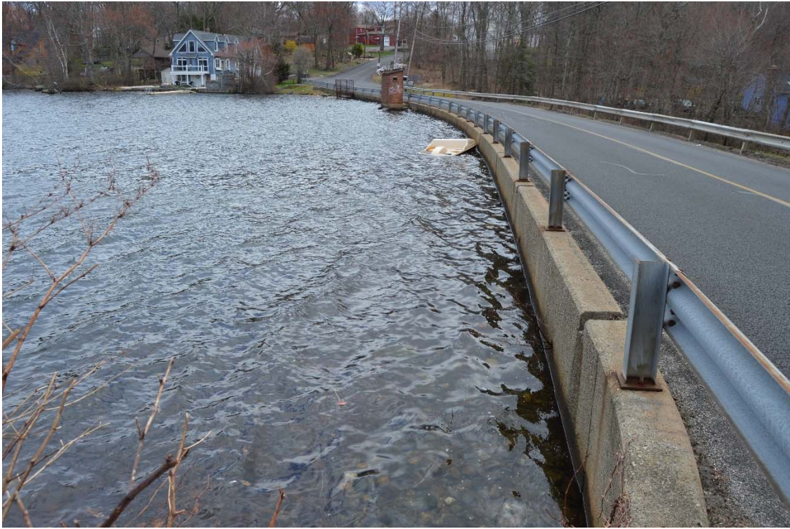
Photo 3a – The upstream side of Cedar Lake Dam, taken from the right abutment area.
