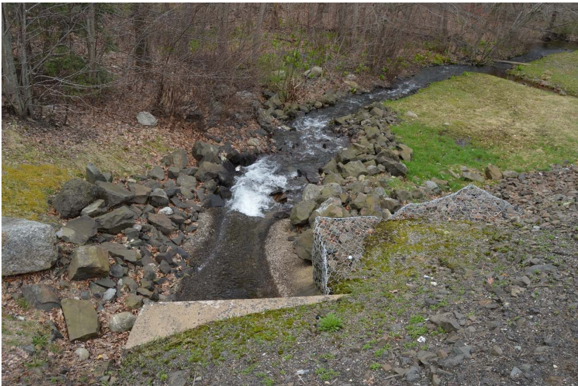
Photo 15b – The upper section of the discharge channel, exiting the spillway tunnel outlet. The riprap along the sides of the channel is stable and generally clear of vegetative growth.
