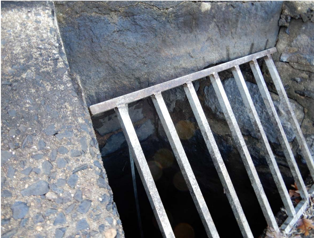
Photo 19i – A close up view of the trash rack at the low level intake, taken during the low water level period in the fall of 2019.
