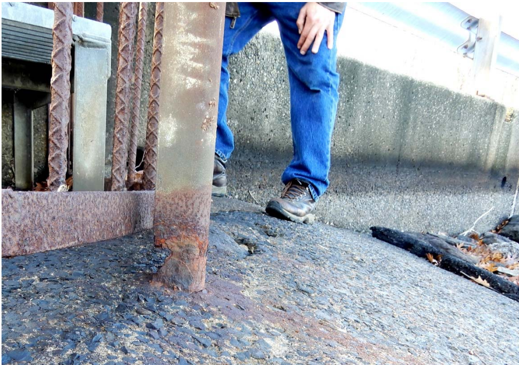
Photo 21r – The base portions of the vertical fence support posts around the upstream spillway approach area are badly deteriorated.
