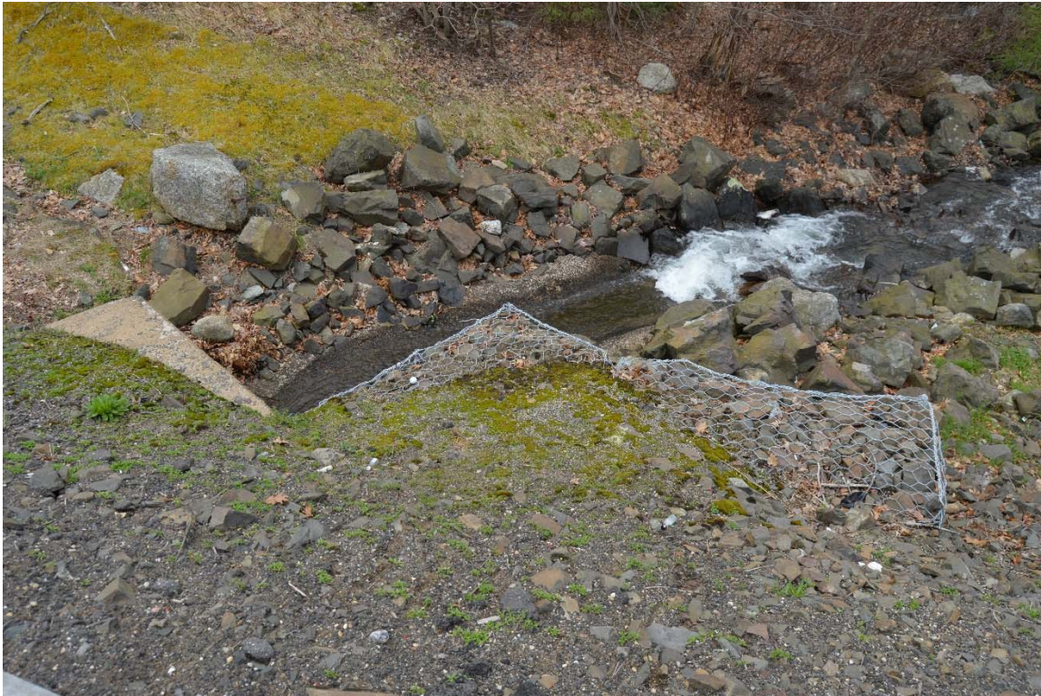
Photo 8b – In the top left corner of the photo is visible the toe of the left-most section of the downstream embankment, east of the spillway outlet channel. Note gabion placement for slope stability at the right side outlet of the spillway discharge tunnel beneath North Street (see also next photo).
