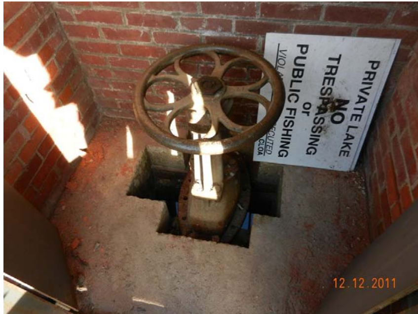
Photo 7: Gate Control for Low Flow Outlet
