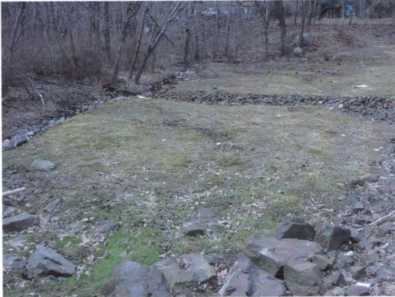
Photo 5 - The left downstream toe area. Note the swale (in the center of the photo) developing from redirected flow emanating from the spillway discharge channel.
