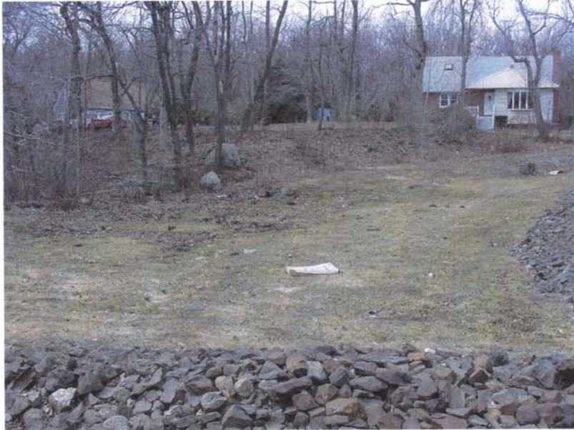
Photo 11 - The right downstream toe area of the dam as seen from the low level outlet channel. The end discharge of the Town's drainage pipe is visible at the center of the photo, as is the saturated groundwater area in the foreground.
