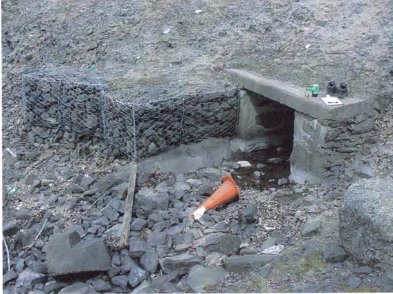
Photo 3 - The downstream discharge from the primary spillway, showing the buildup of debris and riprap in the discharge channel. Due to the rocks blocking the channel, flow is currently directed along the base of the gabions and the left downstream toe of the dam embankment.
