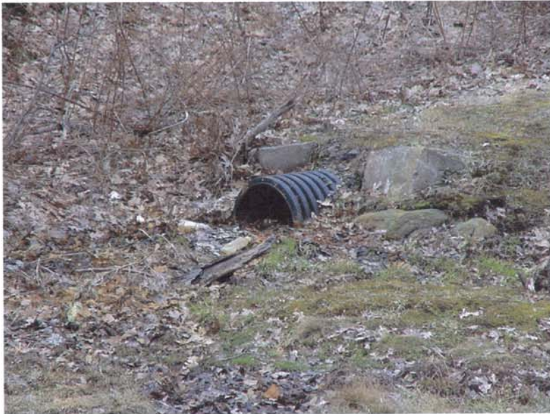
Photo 12 - The discharge of the drainage pipe shown in Photo 11; note that the pipe is partially filled with sediment.
