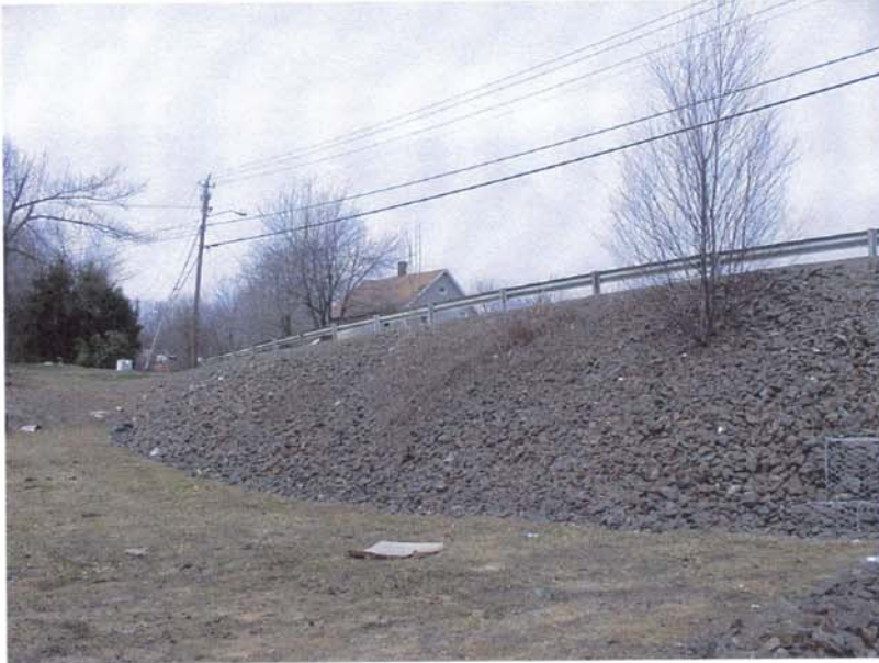
Photo 7 - The right downstream embankment as seen from the low level outlet discharge channel, showing the tree and brush growth on the embankment.
