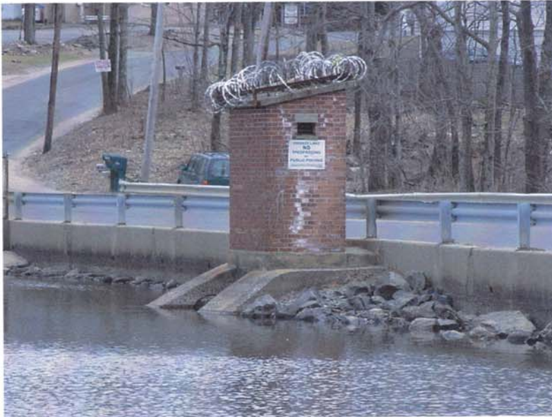
Photo 16 - The gatehouse for the low level outlet at the upstream center of the dam, as seen from the right upstream abutment area.
