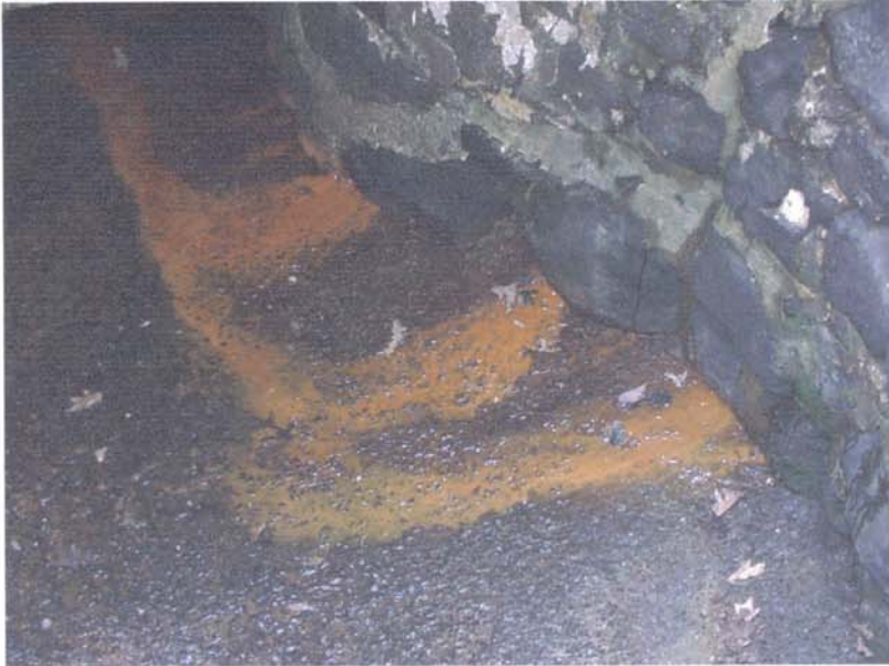
Photo 25 - A close-up view of the seepage at the base of the spillway wall . The seepage is currently minor, but should be monitored on a continuous basis for any change in quantity or quality (turbidity) - as with that noted for the low level outlet discharge area.
