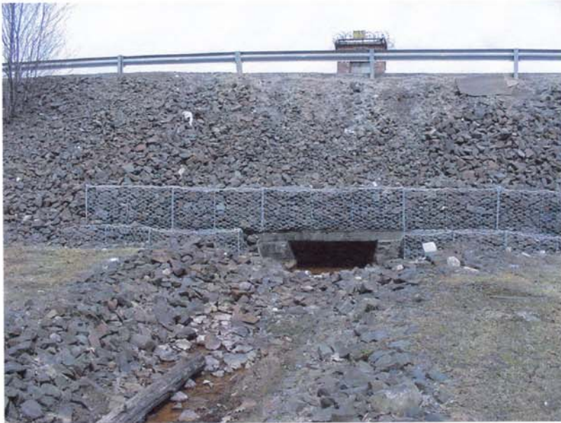
Photo 6 - Looking upstream toward the low level outlet from the upstream gatehouse. Note the good condition of the gabions above the outlet, the erosion and displacement of riprap along the embankment crest and the growth of small trees along the embankment at the left of the photo.
