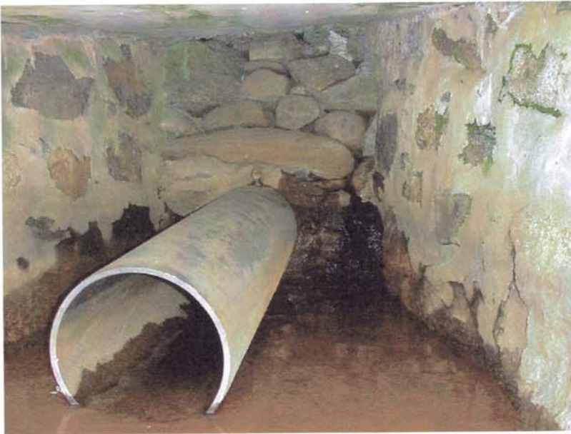
Photo 8 - Seepage emanating from the left side of the low level outlet pipe. The seepage flow rate is currently low, but should be monitored on a frequent basis for any change.
