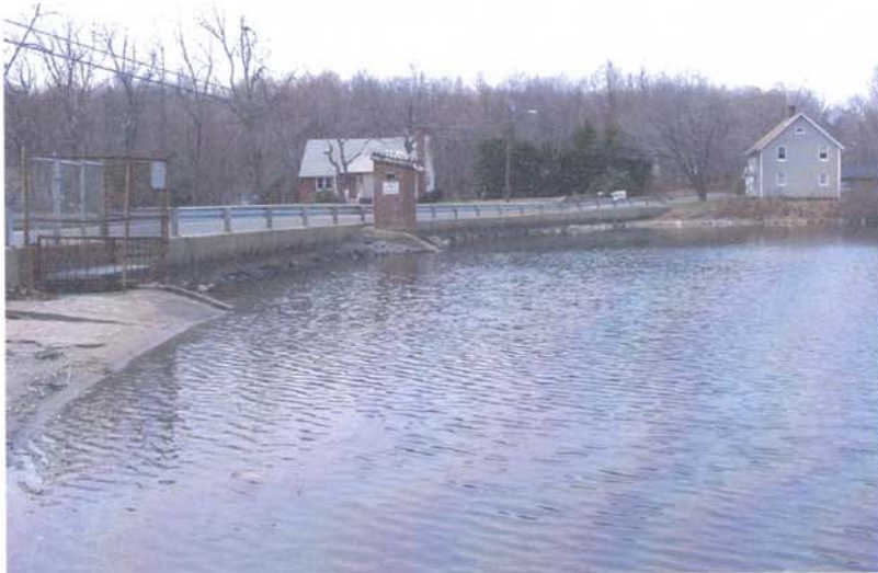
Photo 26 - An overview of the upstream side of the dam as seen from the left abutment area.
