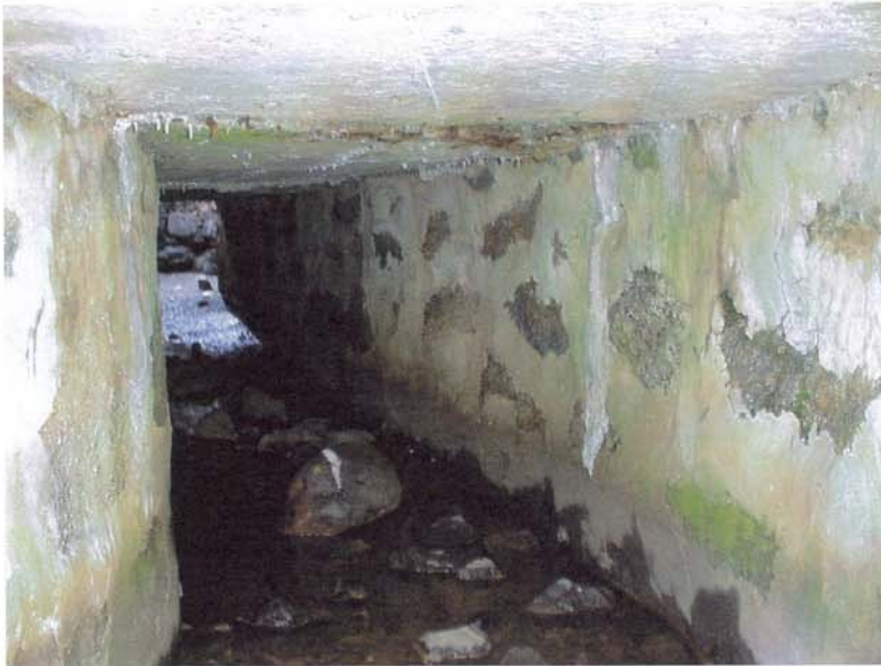
Photo 4 - The inside of the primary spillway discharge channel, looking in an upstream direction. Several large rocks within the "tunnel" are visible along the base of the channel. Note that the overall condition of the channel near the downstream end is good, with sidewalls and roof in relatively good condition (stone and concrete).
