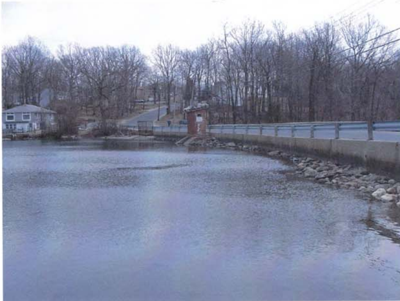
Photo 14 - An overview of the upstream side of the dam from the right abutment. The low level gatehouse is at the center of the photo with the primary spillway just beyond and to the left. Riprap along the base of the upstream concrete wall is in overall good condition.
