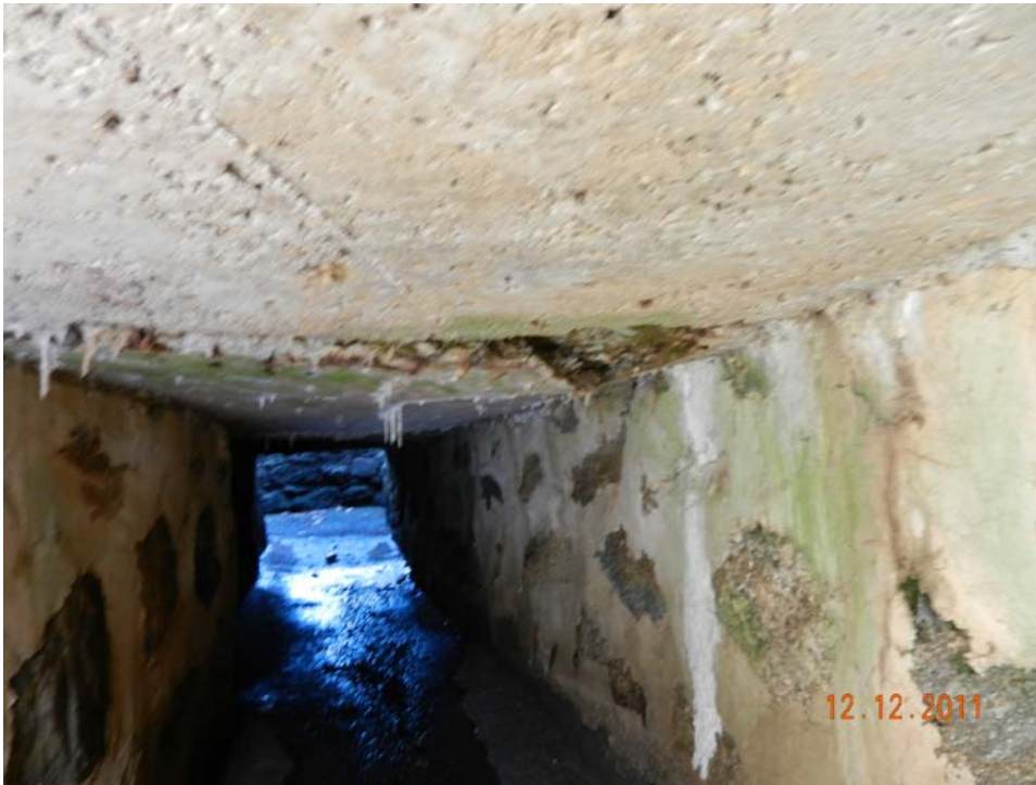
Photo 22 – The spillway discharge tunnel beneath the road, with severe concrete roof deterioration, evidenced by a downward bulge and exposed interior disintegrating concrete.
