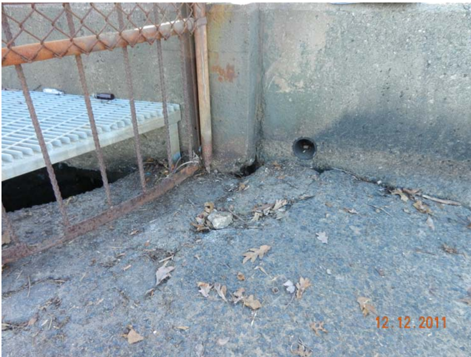
Photo 14 – The right side of the spillway slab, again showing cracked sections of concrete and a void area at the base of the wall. Note also the corrosion of the metal protective barrier, indicative of other sections (see previous photos).
