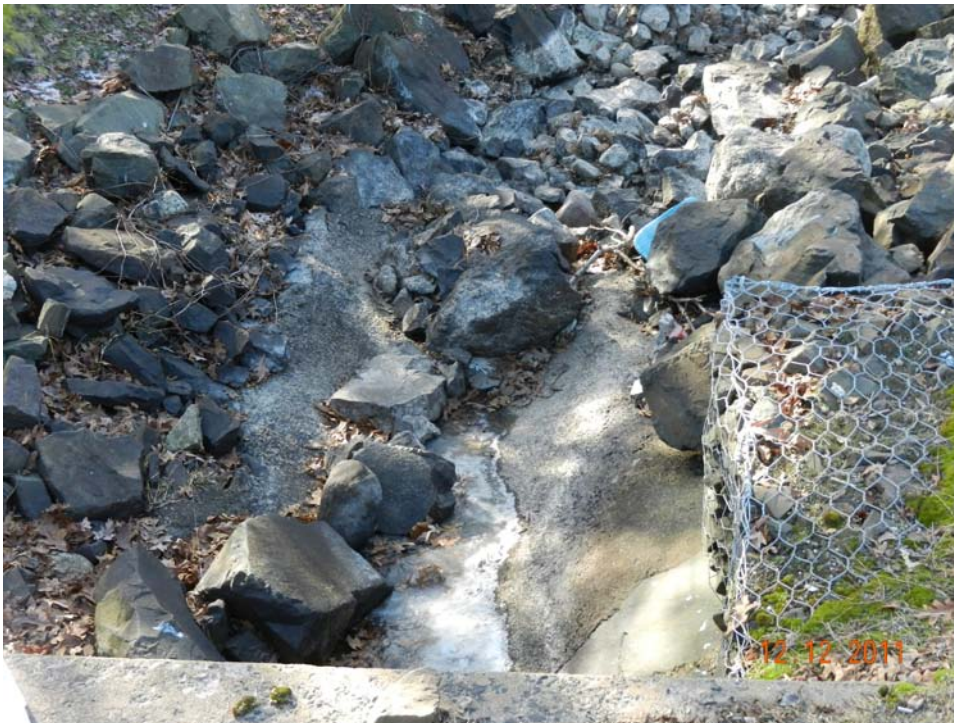
Photo 26 – The existing discharge area for the spillway tunnel beneath the road. Large stones are a partial block to flow efficiency at this channel location.
