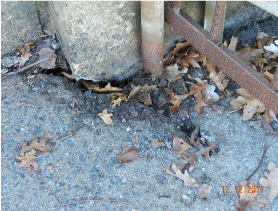
Photo 13 – A closeup of the void area beneath the embankment wall just left of the spillway opening.
