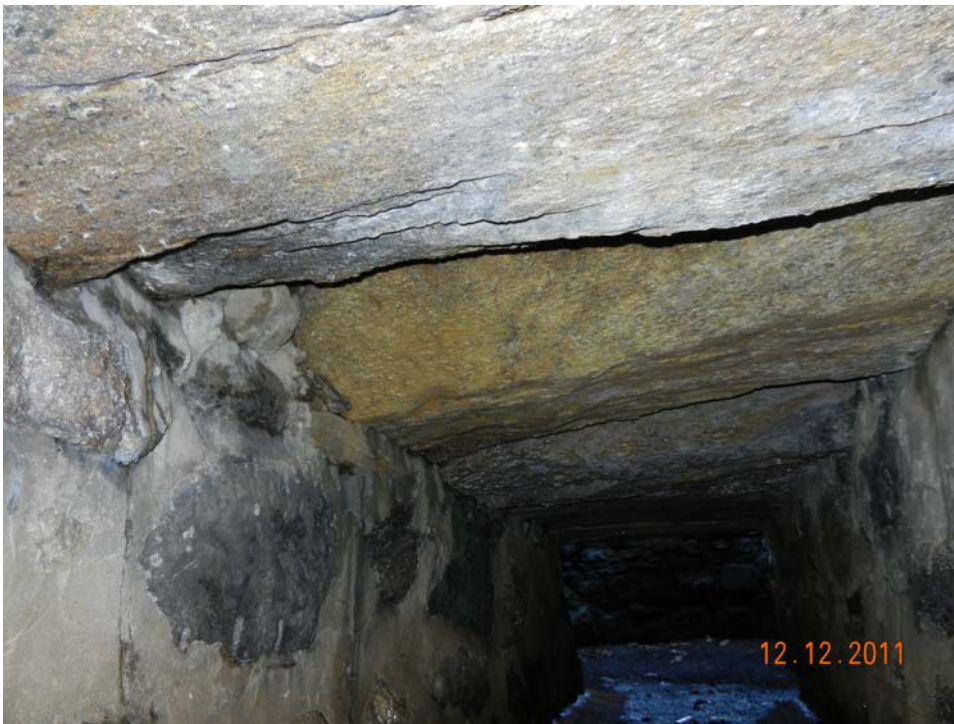
Photo 24 – The roof of the spillway discharge tunnel just beyond the concrete section, at the approximate center of the road above. Note open areas between large stones spanning the structure.
