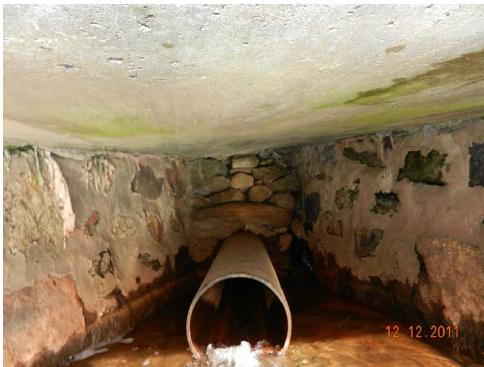
Photo 28 – The low level discharge pipe emanating from the center base of the downstream embankment. This area has changed little since the last inspection and seepage at the wall adjacent to the pipe remains constant.
