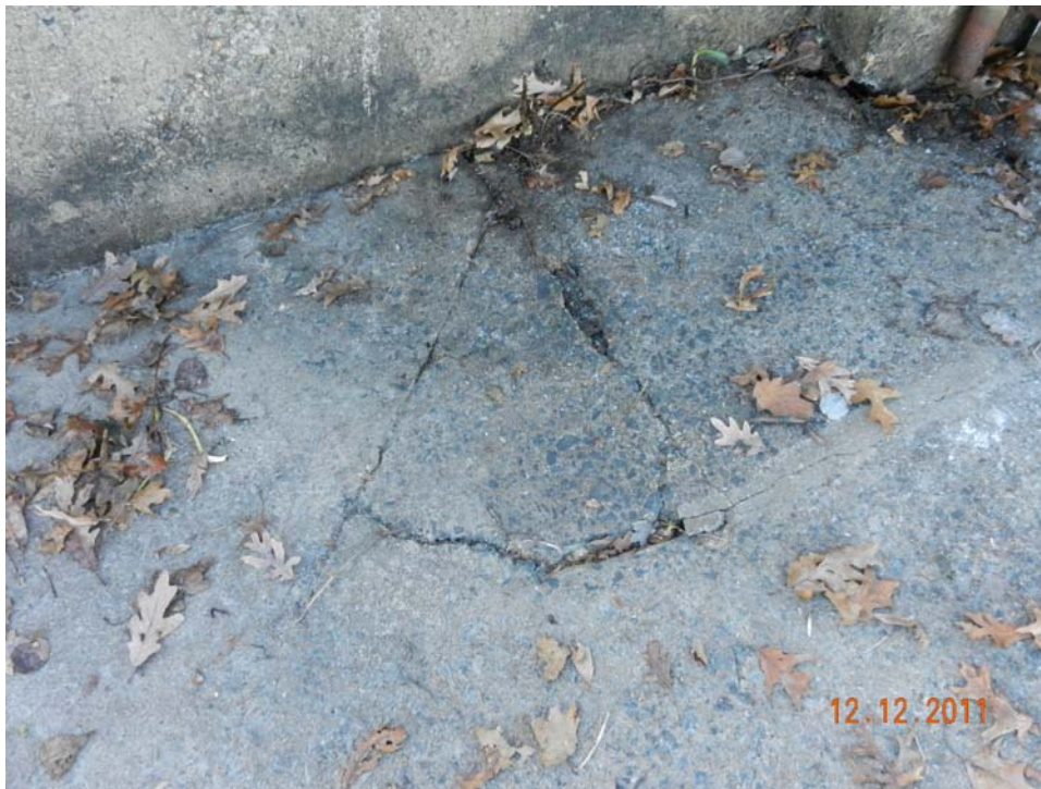
Photo 12 – Cracked section of concrete surface on the left side of the spillway.
