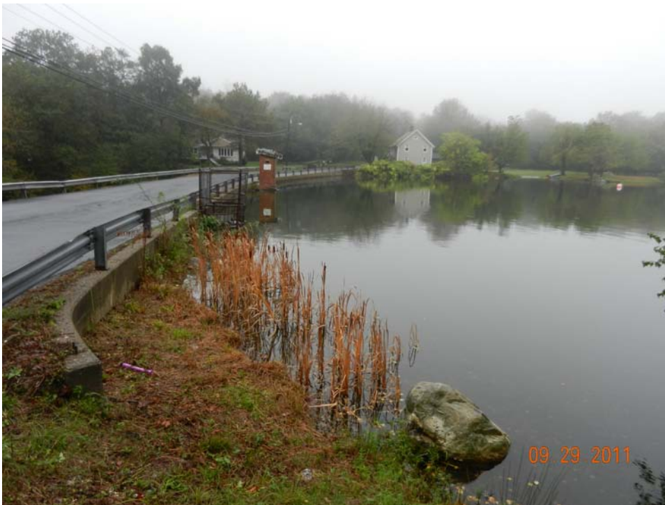
Photo 4 – The left upstream end of the embankment showing vegetation along the wall area to the left of the spillway.
