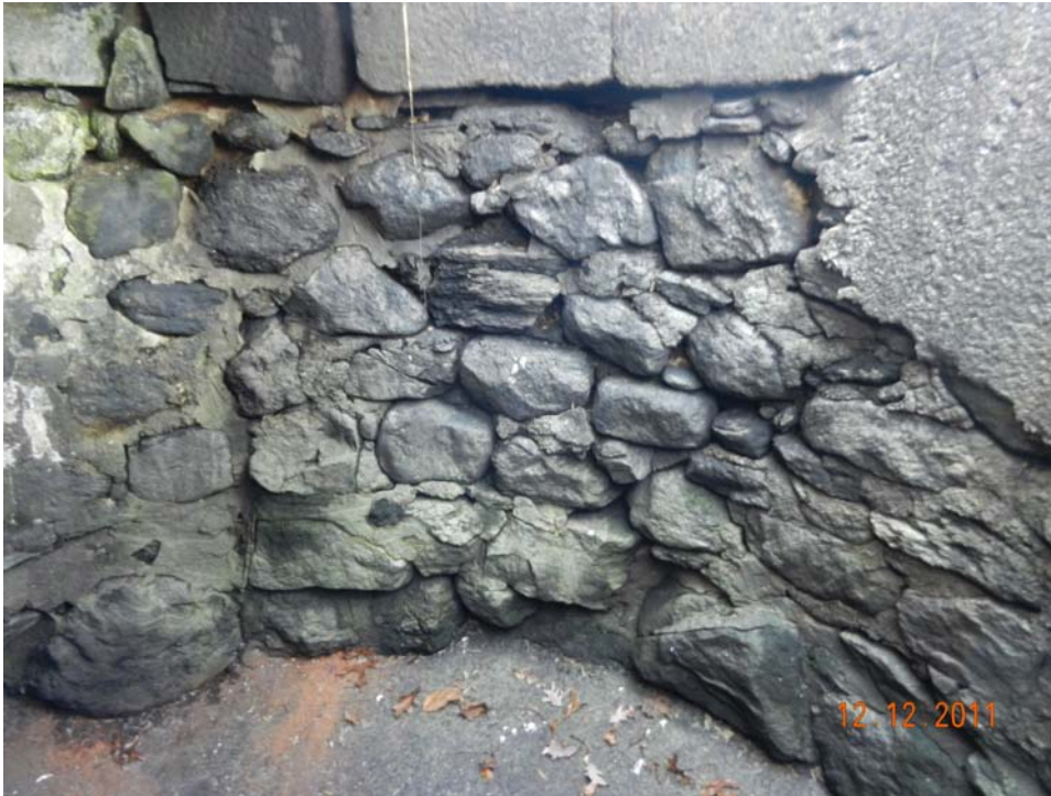
Photo 25 – Interior of the spillway drop structure, showing some of the smaller typical voids in the stone wall and the staining from seepage and leakage at the base. A note for Photo 15 shows that some of this seepage may be from a void at the spillway slab and wall juncture area at the top of this wall.
