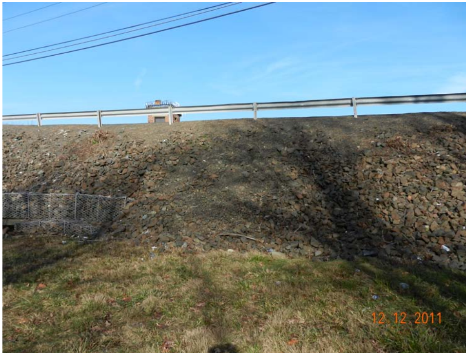
Photo 27 – A portion of the downstream slope showing an area of surficial sloughing caused by the steep slope and the movement of pedestrians along the top crest behind the guard rail.
