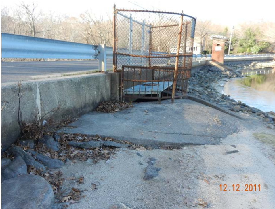
Photo 11 – A view towards the spillway. Note the woody vegetation growing at the base of the vertical joint at the left of the photo and the crack along the concrete surface in the center.
