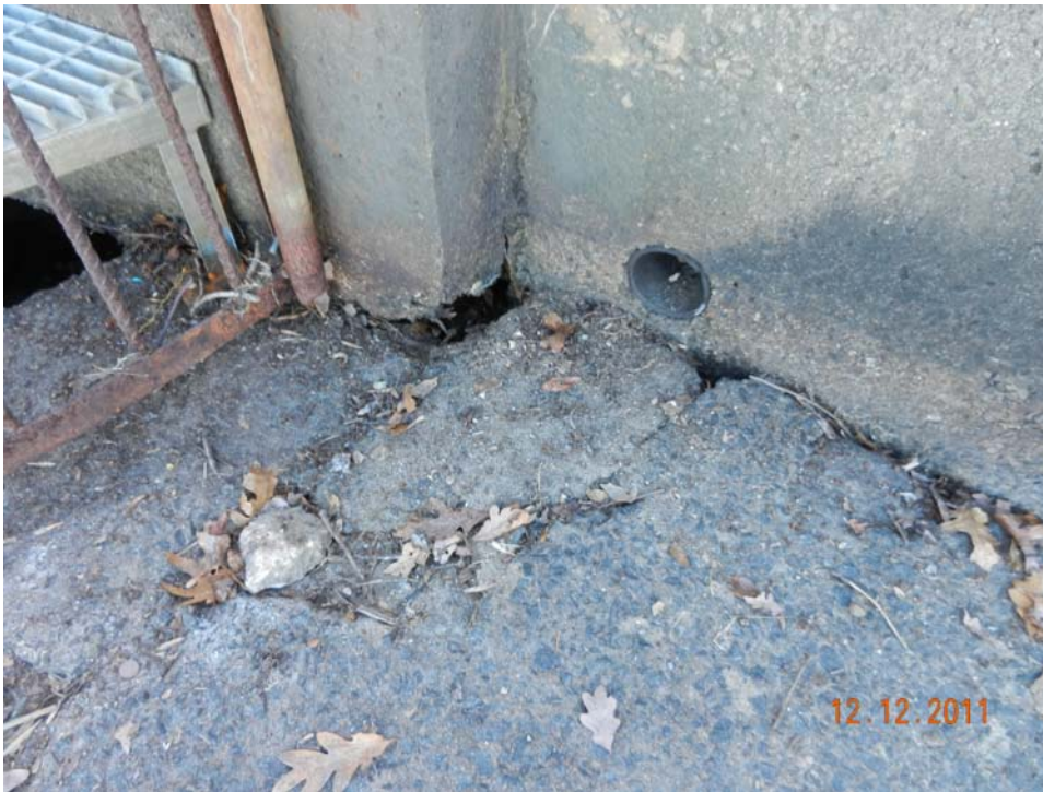
Photo 15 – A closeup of the view of the void area beneath the wall in Photo 14; this void went at least 9” deep beneath the wall and is very likely the source of some of the seepage emanating from the base of the masonry wall beyond.
