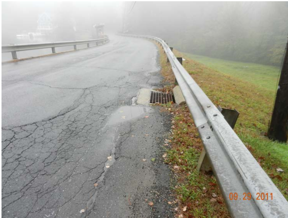
Photo 9 – A rutted and cracked asphalt area near the right end of the dam, indicative of many of the other asphalt issues along the top of the embankment.
