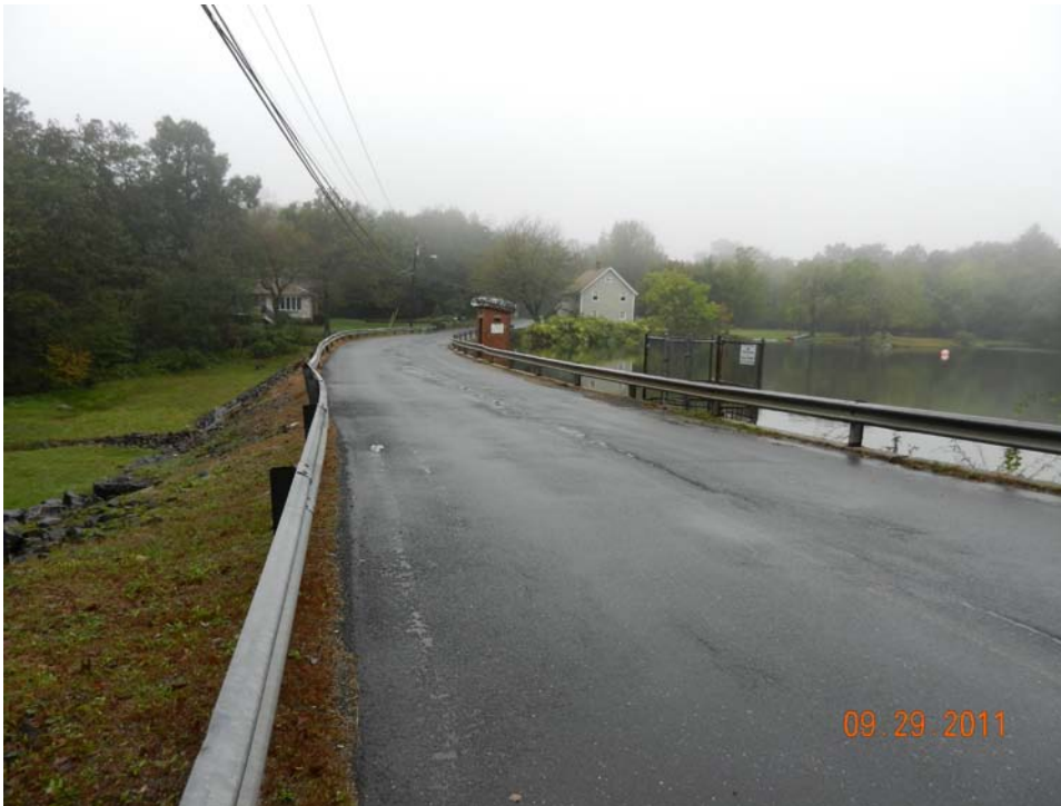
Photo 3 – The roadway forming the top of the dam embankment, looking westerly from the left side.
