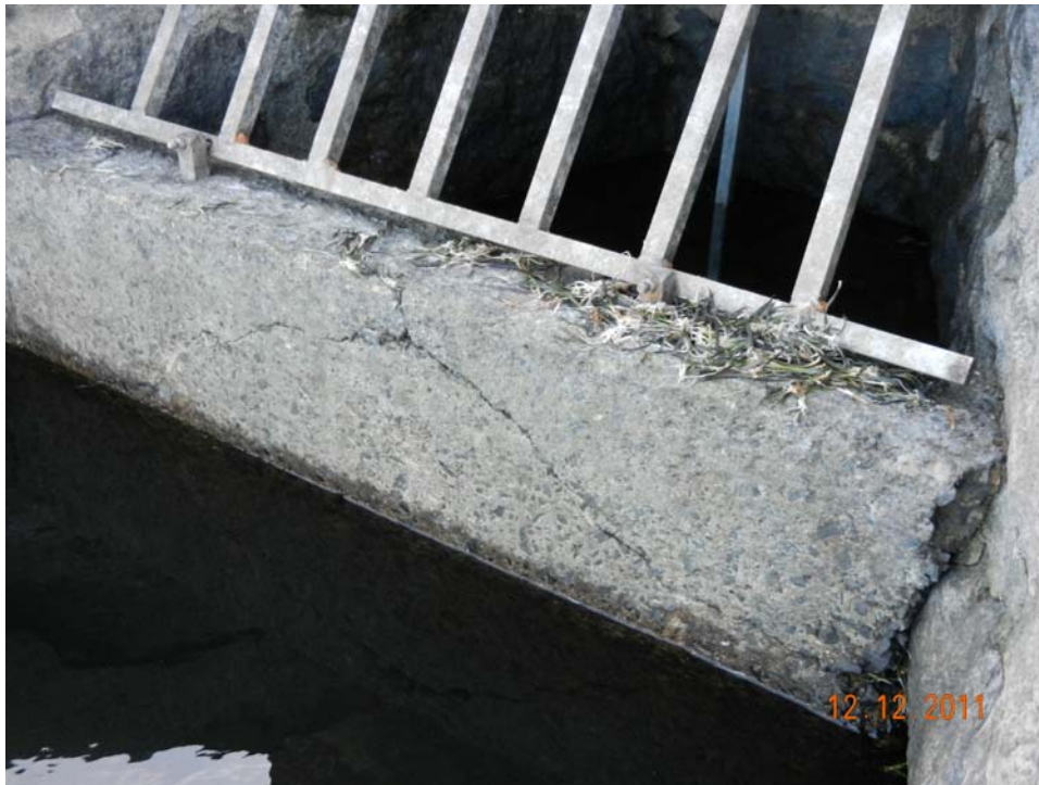
Photo 17 – A closeup of the trash rack support at the gatehouse intake, with a 30” long crack and a broken section adjacent to the wall.
