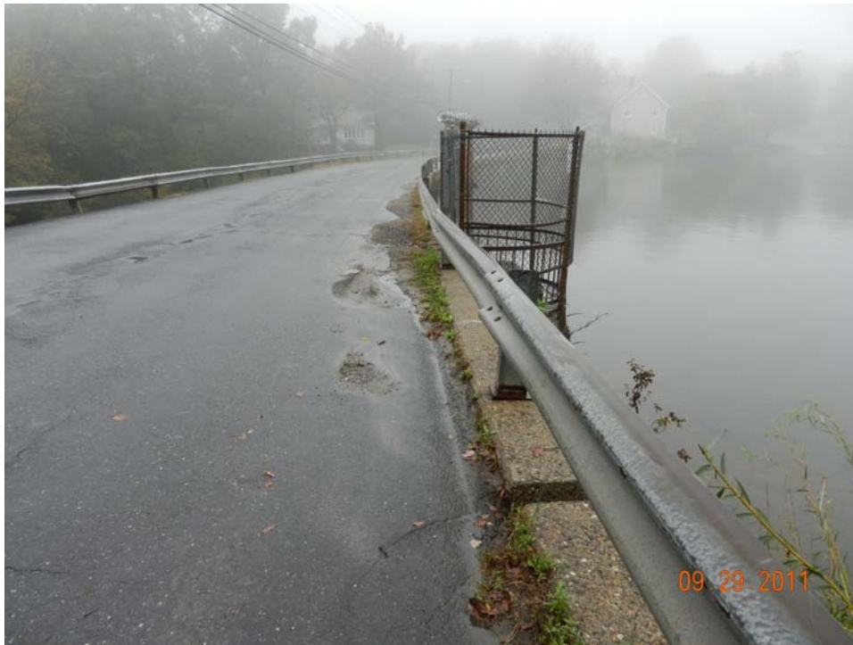
Photo 7 – Looking westerly along the top of the dam and roadway toward the spillway overflow at the center of the photo. Note the sediment deposits along the edge of the road and top of wall where there is periodic ponding.
