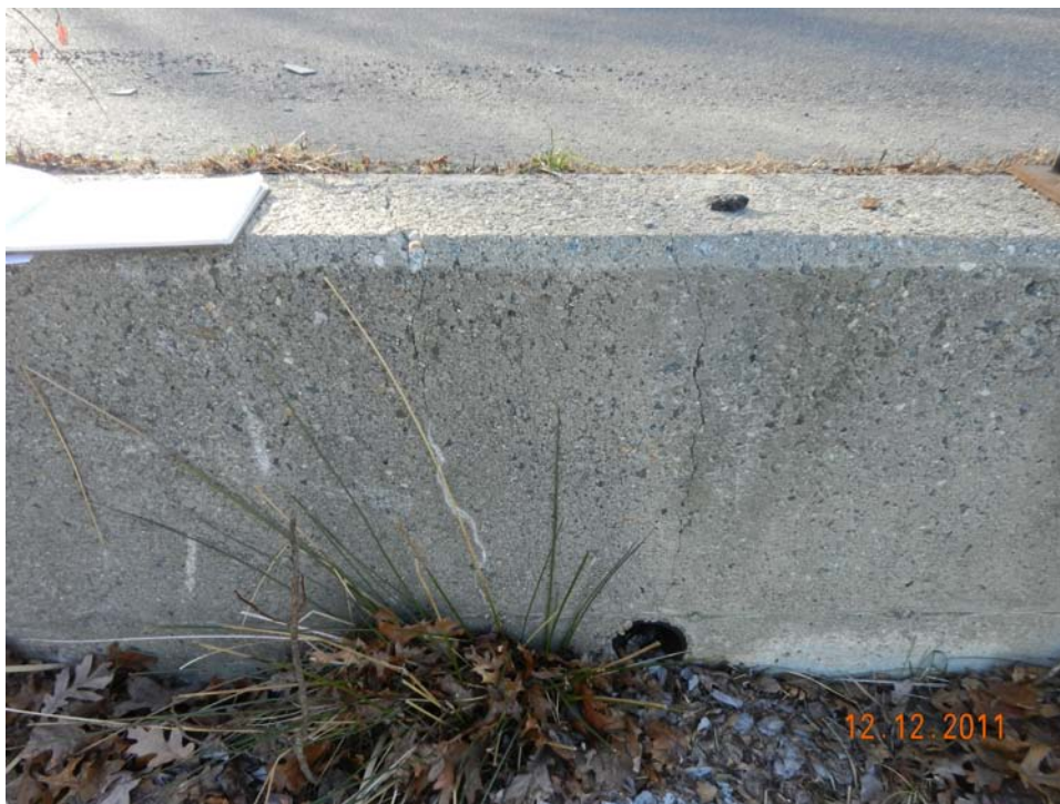
Photo 10 – One of the many minor vertical cracks along the upstream concrete embankment wall that needs to continue to be monitored.
