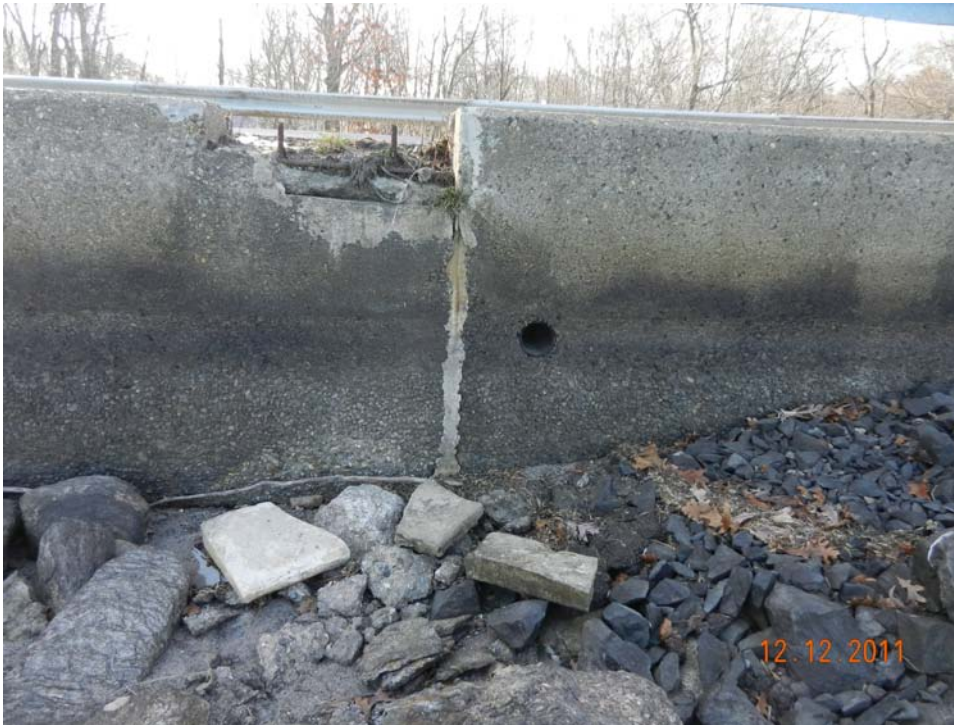
Photo 16 – One of the many vertical joints with deteriorating sealant. This one has vegetation growing out the top, with sealant being pushed out by the roots.
