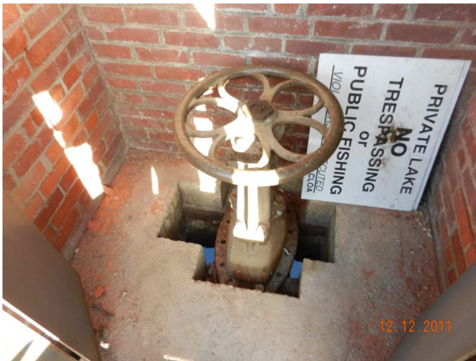
Photo 18 – Interior of the gatehouse. Note the mild corrosion on the gate wheel control mechanism and some spalling of interior brick (see chips at left base).
