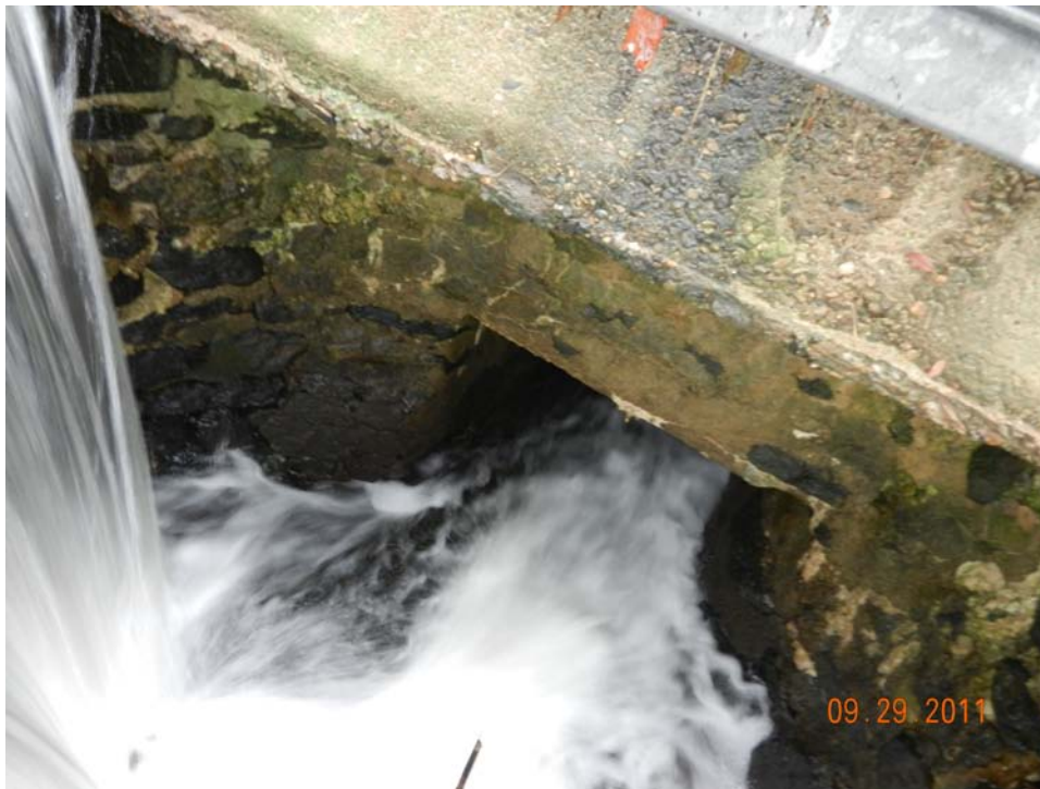
Photo 6 – Flow over spillway dropping into the entrance area of the tunnel / culvert beneath the road.
