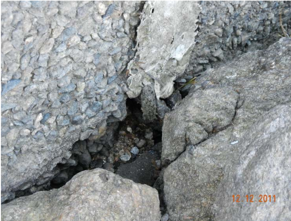
Photo 19 – Typical of the vertical expansion joints is the missing sealant at the base and open voids leading beneath the wall. Footing conditions are unknown at these locations.
