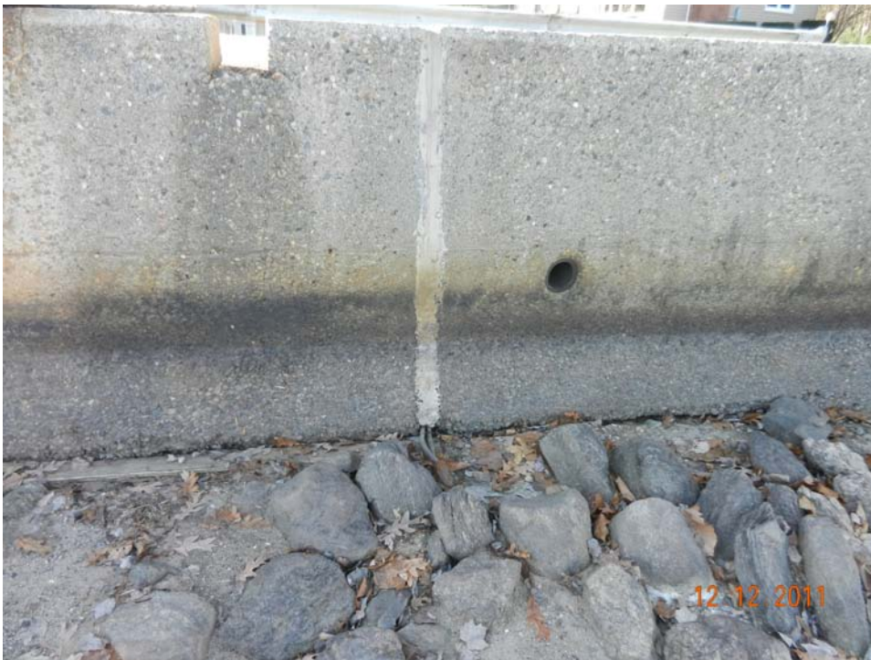
Photo 20 – Another of the vertical joints. Note that at this location, the void at the base of the wall extends on both sides for a total length of about 5' to 6'.
