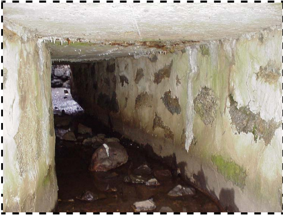
Photo 23 – Comparison photo from the 2006 inspection showing the interior condition of the discharge tunnel area. Note the difference in roof condition.
